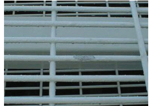
Img. 3.5.6. Uneven surface caused by poor zinc coating
