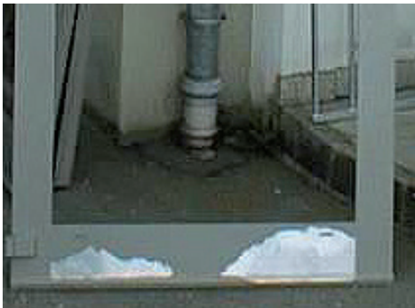
Img. 5.3.4. Blistering caused by an inappropriate pretreatment
