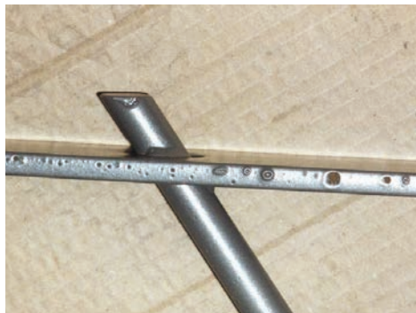
Img. 3.6.2. Bubbles caused by corrosion after pretreatment
