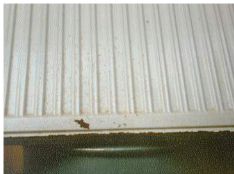
Img. 5.1.2. Infiltration caused by chemical exposure
