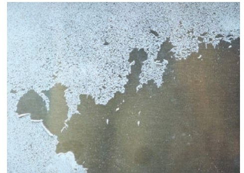
Img. 3.9.3. Insufficient wet out of the substrate
