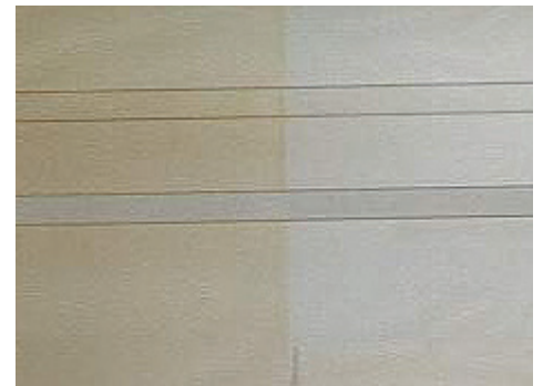
Img. 4.4.3. Yellowing in the interior caused by UV-light
