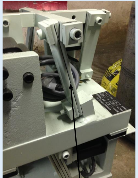
THE SPACE BETWEEN THE SPRINGS CAN TRAP DIRT AND DEBRIS
