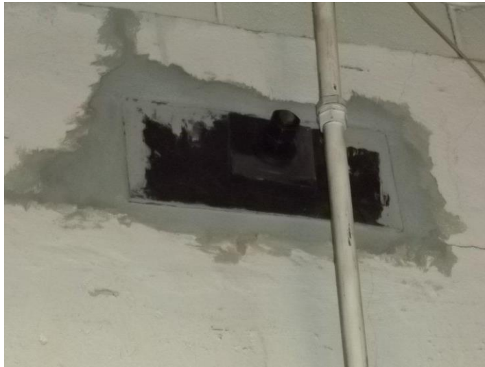
Figure 62: Firefighters should maintain situational awareness and report if they observe a cable and/or plate on the exterior wall. This can be an indicator of bowstring truss or a repaired roof structure.
