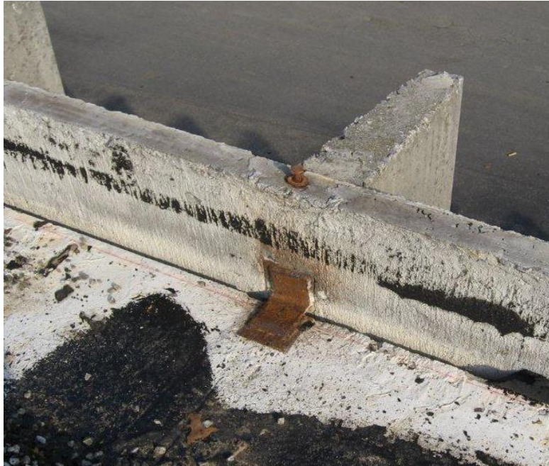
Figure 47: Note the metal connector connecting the roof and exterior, tilt up wall.
