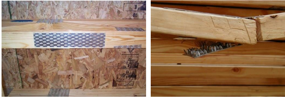
Figure 32: Truss connectors before and after partial collapse.
