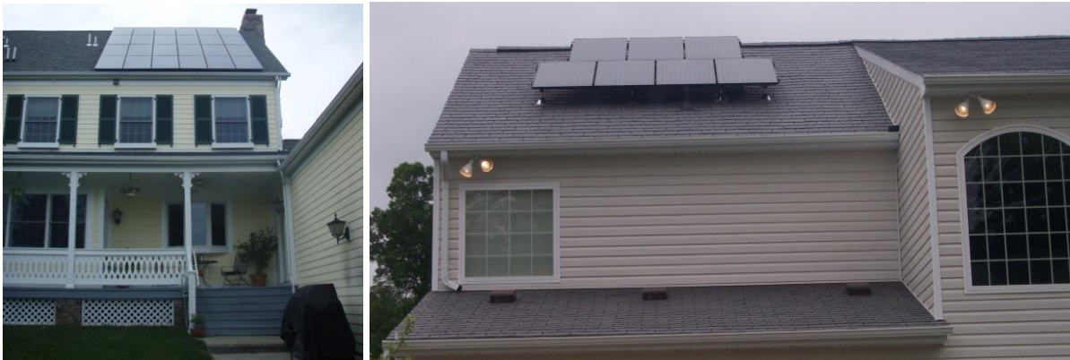
Figure 69: Typical Solar arrays for residential application.
