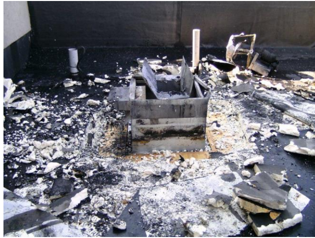
Figure 31: Grease fires often extend upward into the roofing materials.
