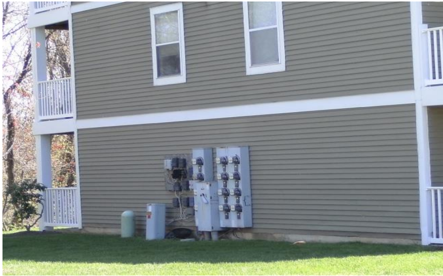
Figure 30: The location and control of utilities is an important function of the truck company.
