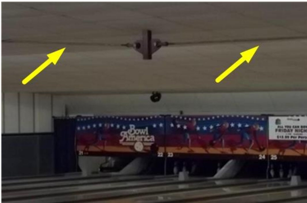
Figure 61: Ceiling tiles can hide what would normally be an easy visual clue of a bowstring truss roof. Prior knowledge of these buildings is essential when firefighting fire.
