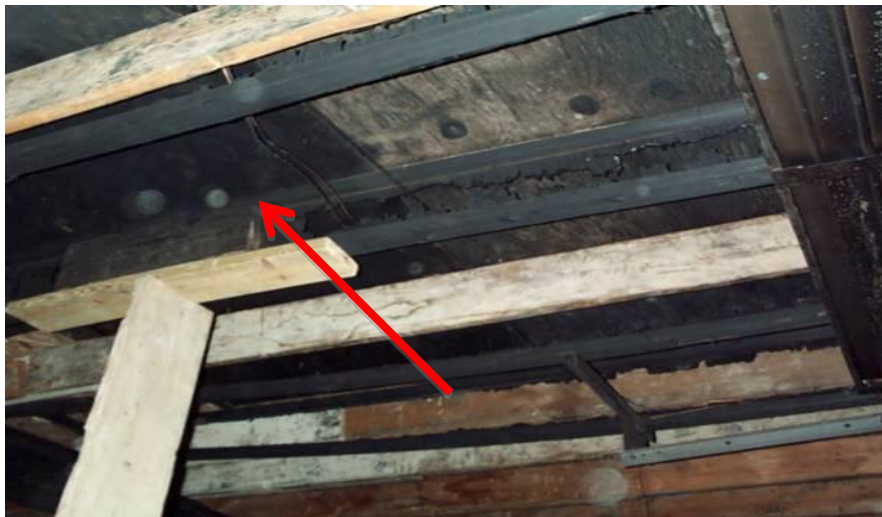
Figure 34: Plywood I-beam subjected to fire conditions and has disintegrated.
