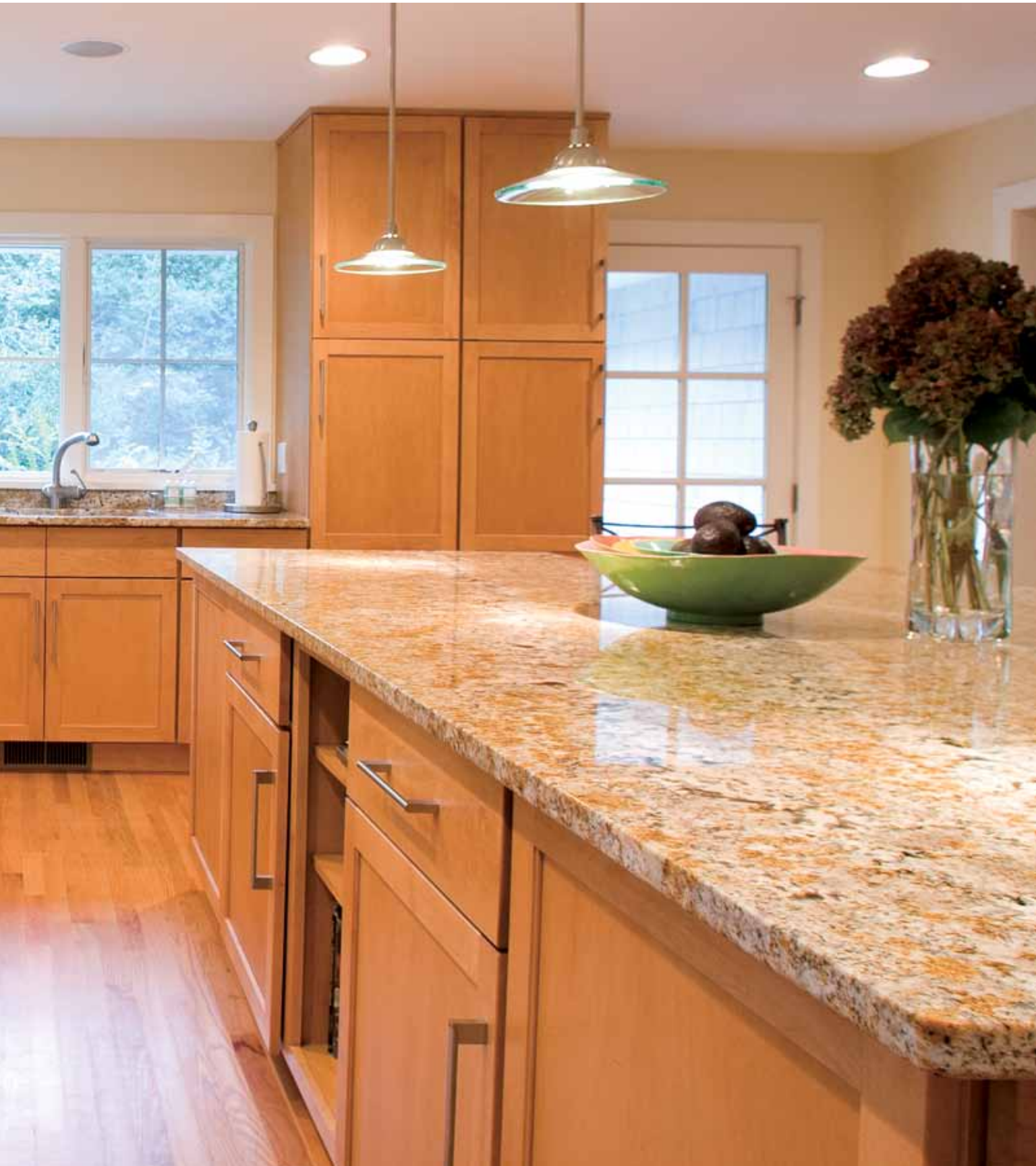
THIS BEACH HOUSE IN AN EXCLUSIVE AREA OF DELAWARE WAS A LABOR OF LOVE FOR THE LYONS, REQUIRING EXTENSIVE RENOVATION.
