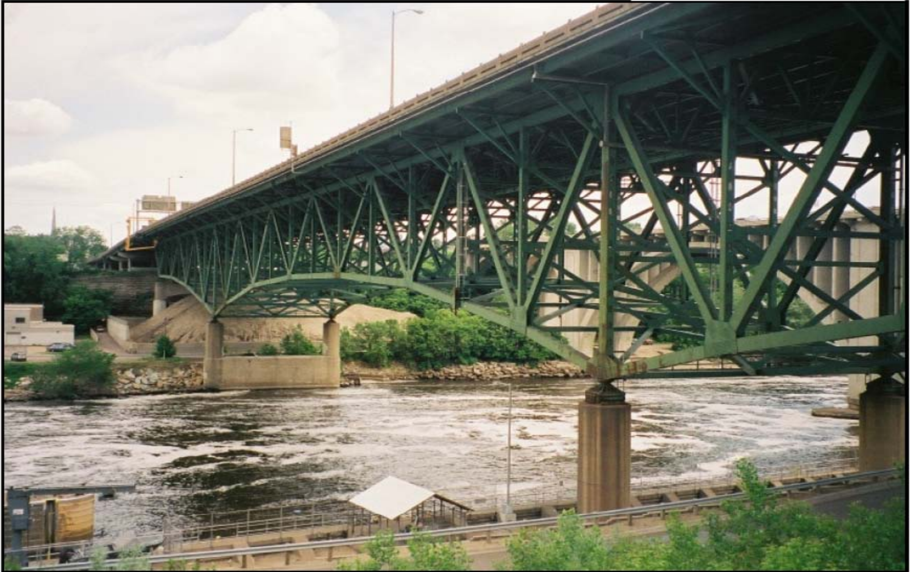
A view of the west side of the deck truss portion of the bridge, looking northeast.
