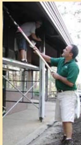
Steve Shively and members of the maintenance crew kept busy this summer. Darin Blume is on scaffold in the background during painting of the Sequoia Building.
