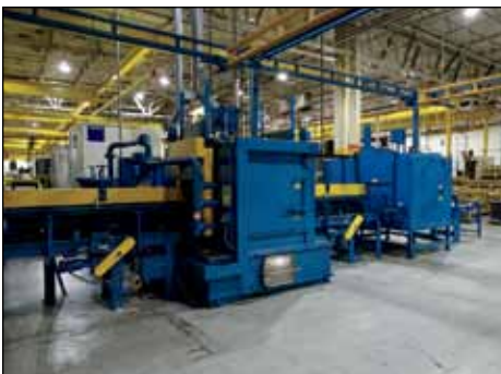
PROCECO AQUEOUS CONVEYORIZED WASH LINE
