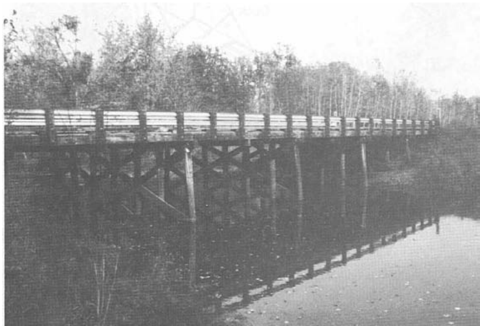
Figure 2-11.- Sawn lumber longitudinal deck bridge. Note the transverse distributor beams attached to the deck underside between bents (photo courtesy of Wheeler Consolidated, Inc.).
