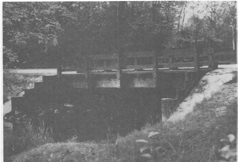
Figure 2-5.- Typical sawn lumber beam bridge. Most lumber beam bridges of this type span 25 feet or less, but longer spans have been built where large beams are available.
