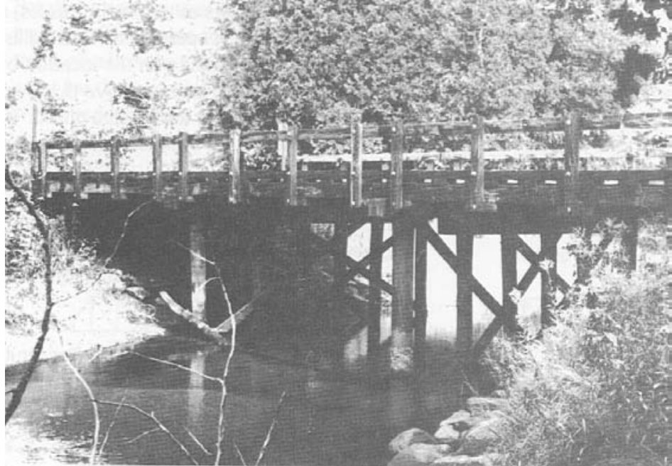
Figure 2-10.- Longitudinal glulam deck bridge over Au Train Creek on the Hiawatha National Forest. This bridge is 58 feet long over three spans and supports a 26-foot roadway width.
