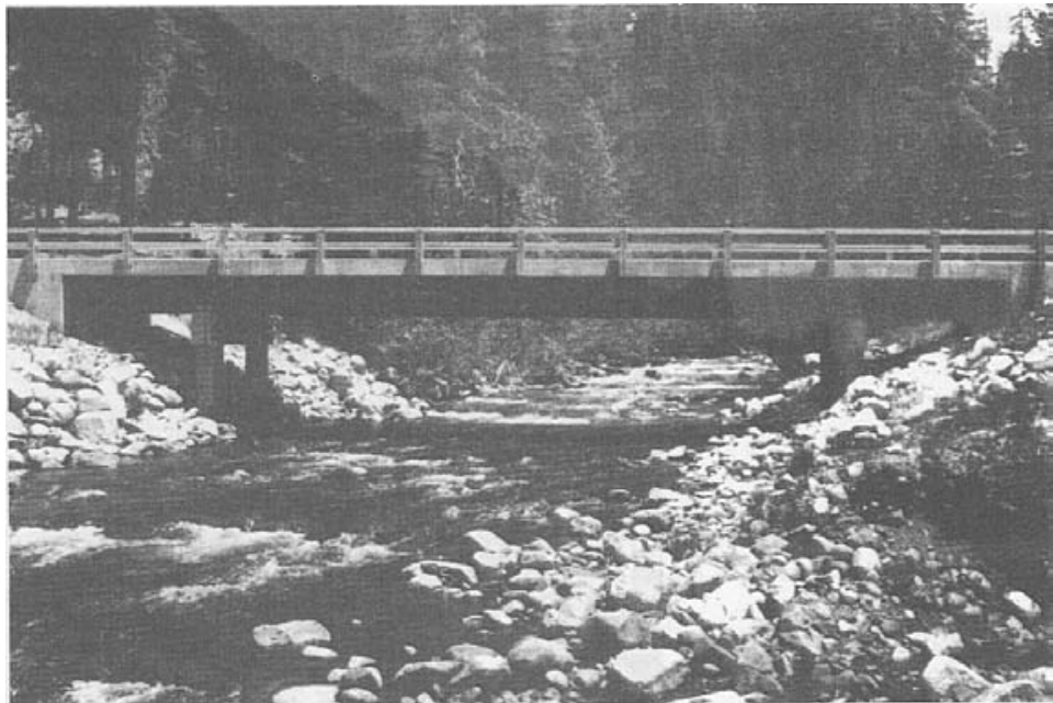
Figure 2-26.- Composite glulam-concrete T-beam bridge located in northern California. Although numerous bridges of this type have been built, they are not common.
