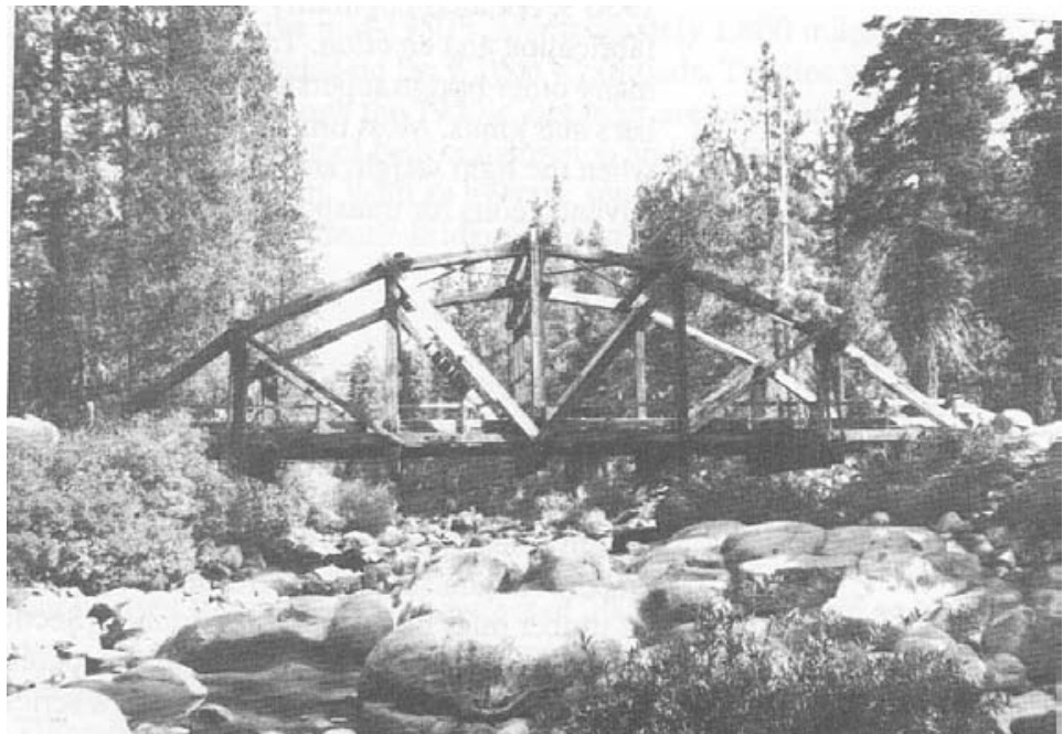
Figure 2-14.- Lumber bowstring truss over Dinkey Creek on the Sierra National Forest in Central California. This truss spans 90 feet and was built in 1934 (photo courtesy of Raul Gonzalez, USDA Forest Service).
