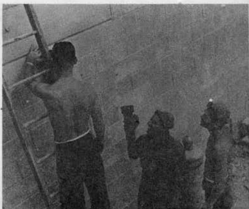
NO HOT WATER - J.W. Smith, UT2; J.A. Falas- ca, UT3, and D.G. Myers, "B" Company men, perform construction of pipe outlet on the AUW Building.
