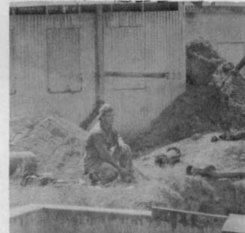
PIPE PATCHING - Taking a break on the POL line site after long hours of pipe patching in the hot sun is P.R. Schroeder, BUCN.
