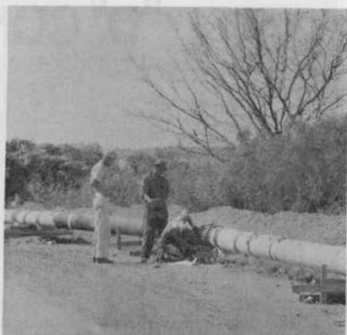
POL LINE CHECKS - Two "C" Company seabees check the pipe on the POL line for breaks and defections.
