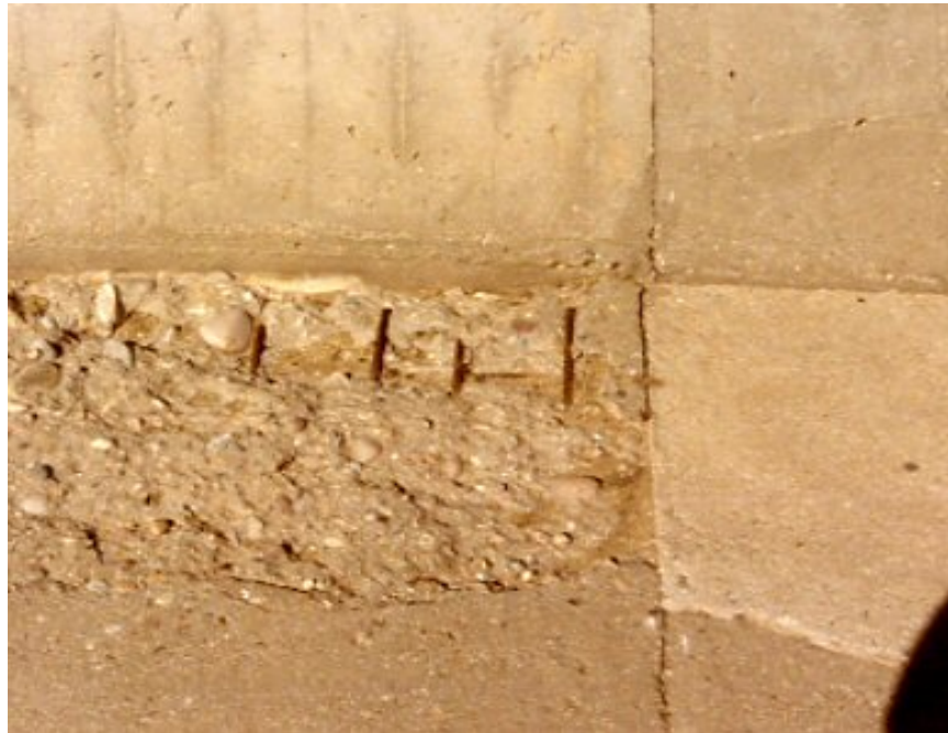
Figure 8. Spalling at Spillway Joint (downstream is toward top of figure)
