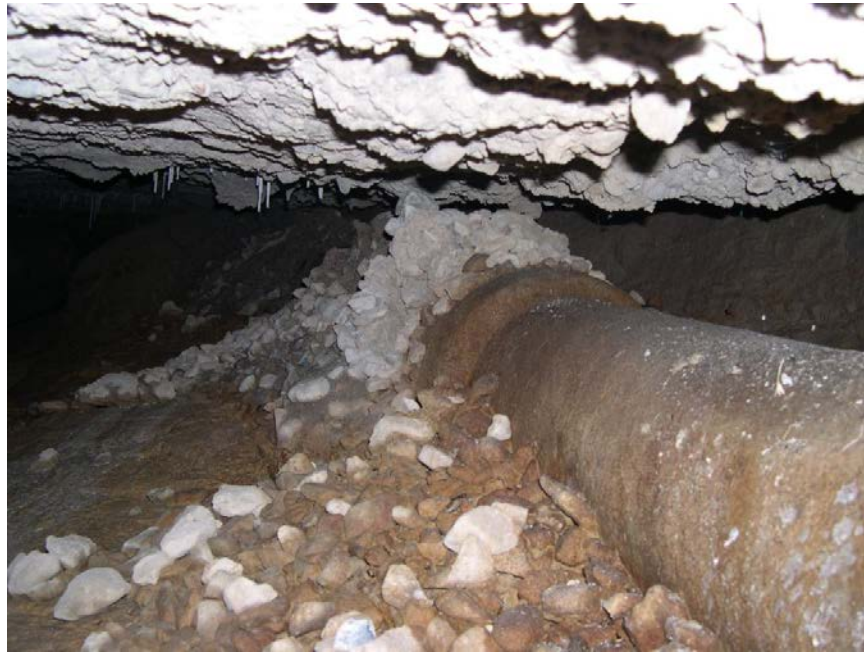
Figure 13. Erosion of Foundation Material Creating Void under Chute
