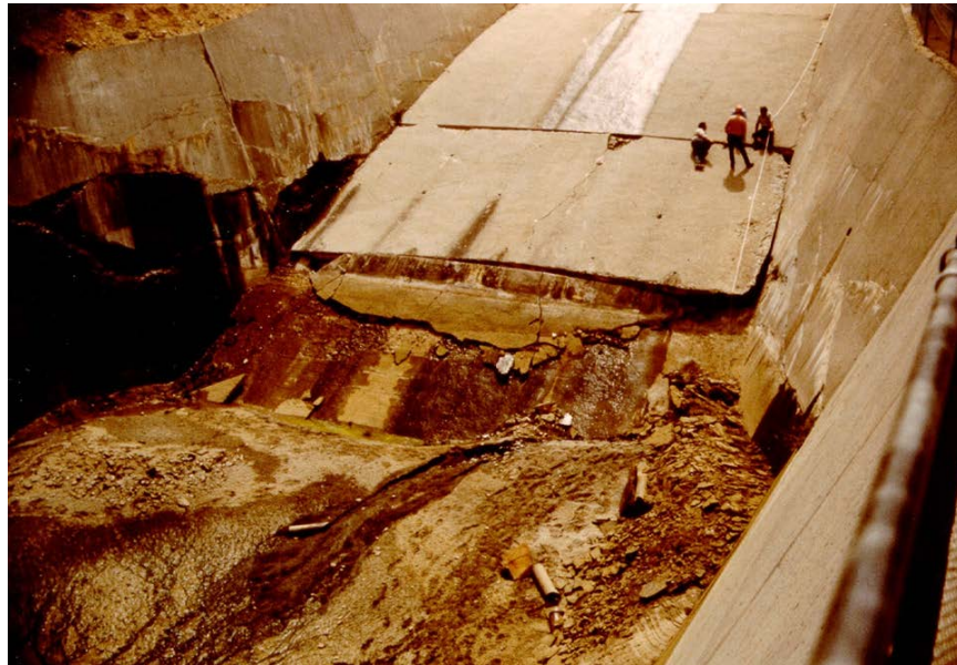
Figure 10. Lost spillway slabs
