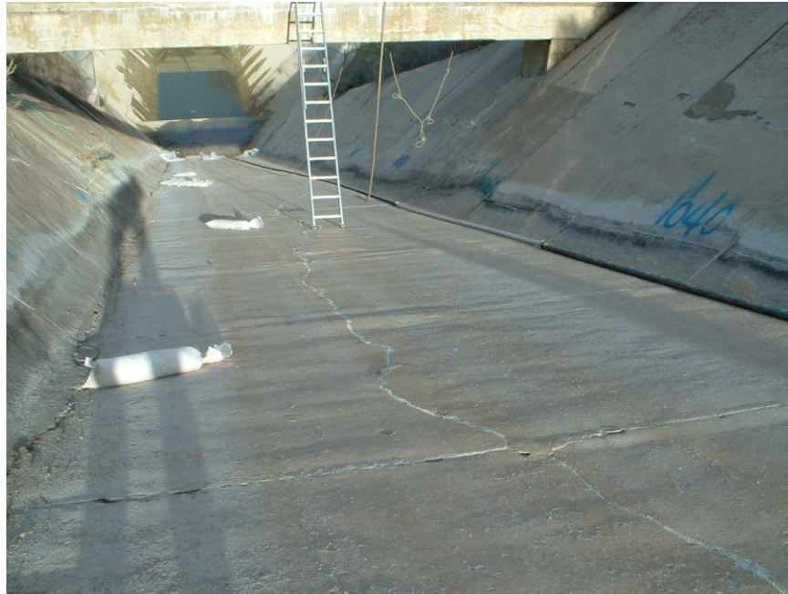
Figure 12. Cracking along the Center and Sides of the Chute Suggest Loss of Underlying Foundation Support
