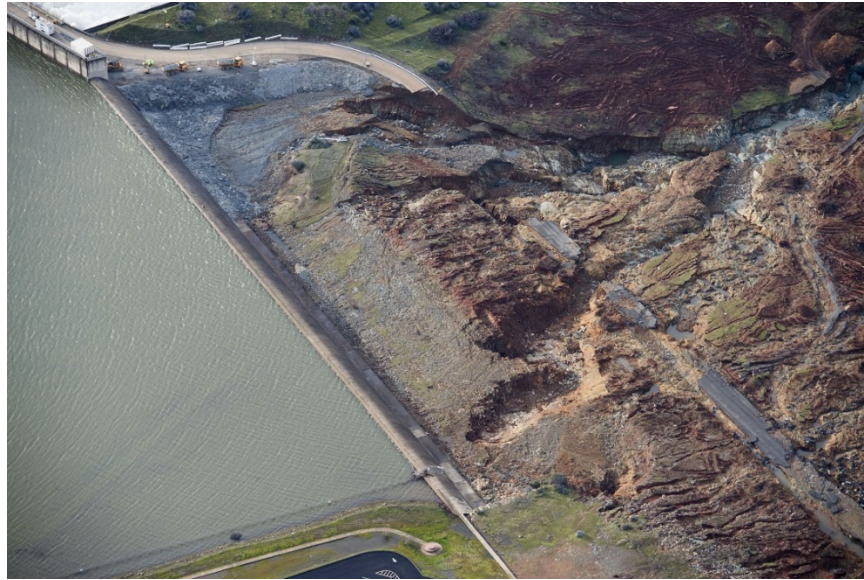
Figure 5. Damage from Releases over Emergency Spillway (the large hole near the right side of the ogee section is downstream of Monoliths 4, 5, and 6)
