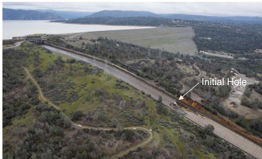
Figure 3. Initial Hole in Spillway Slab
