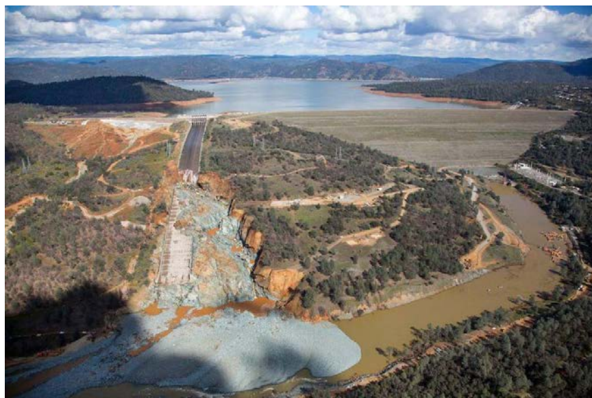
Figure 6. Damage to Service Spillway and Debris Washed into River
