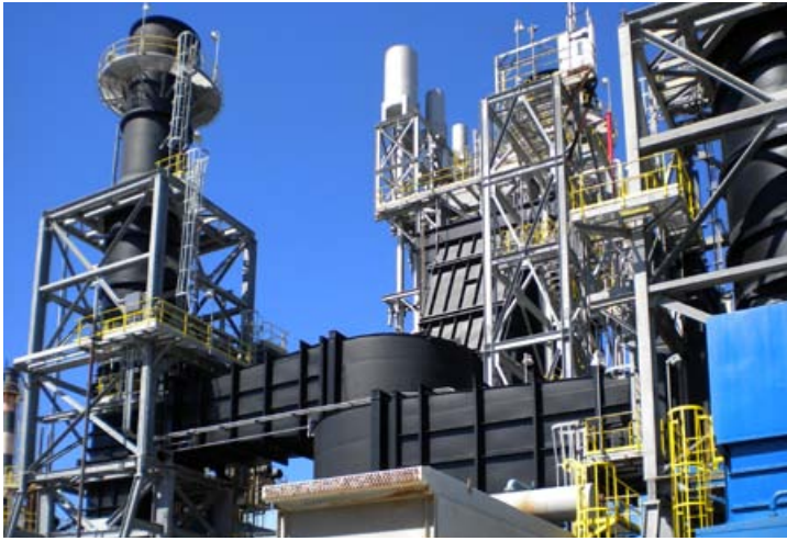
WAPA plant on St. Croix. Photo by Dan Olis, NREL/PIX 18598
