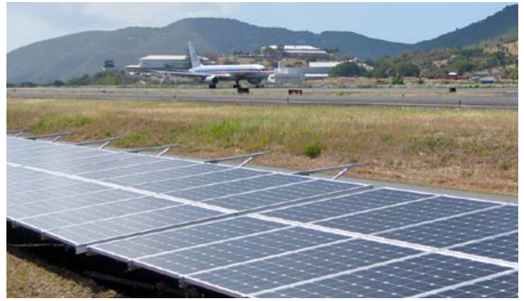
A 448-kW PV system installed at the Cyril E. King Airport on St. Thomas in April 2011. Photo by Adam Warren, NREL/PIX 18953
