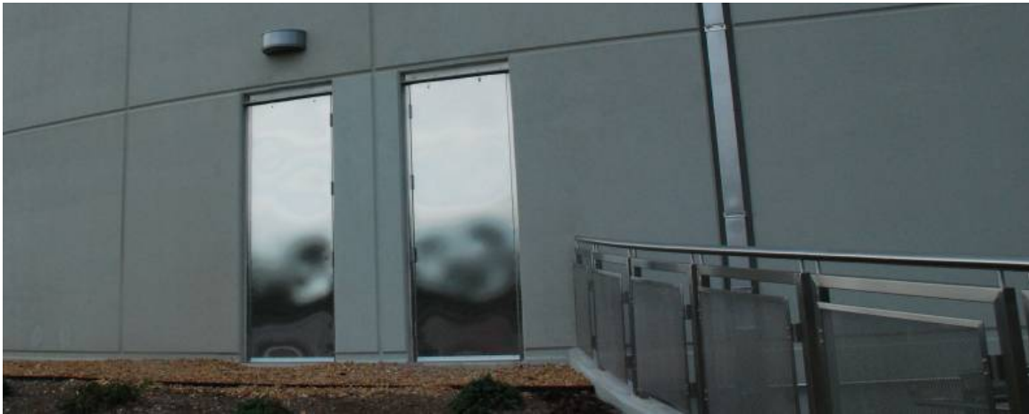
Figure 3-5 Emergency Exit Doors
