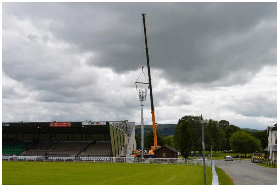
Figure 33: The permanent EE Mast craned into position on the Royal Welsh Showground (June 2016)
