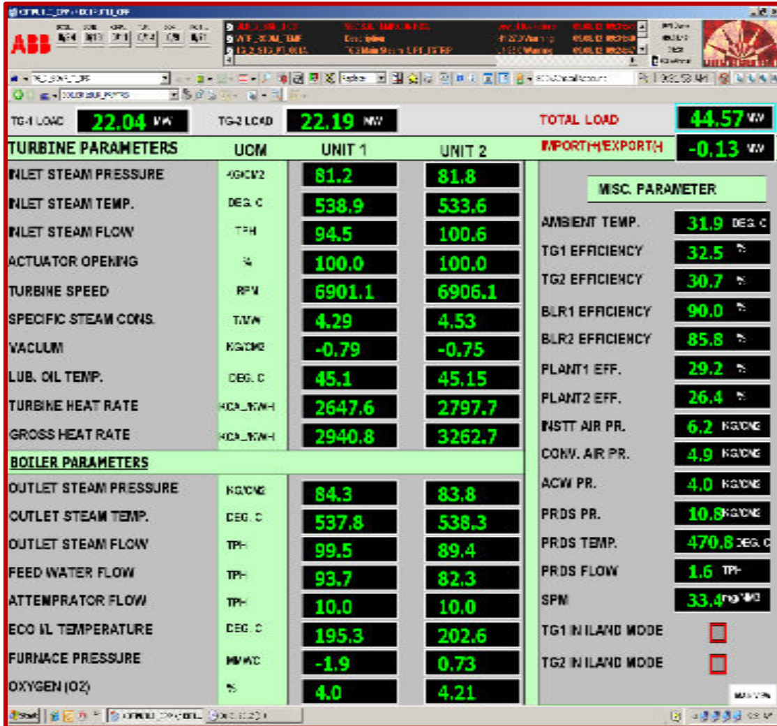
On line Efficiency monitor
