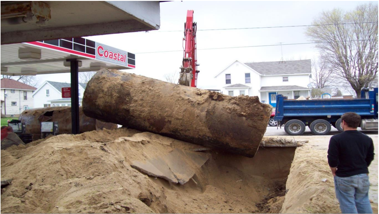
Top photo: Tank removal in Waukon. Planning a tank removal must take into account overhead power lines and canopies that can present risks for removers.
