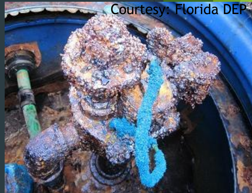
Corrosion on submersible pump head of an E10 tank in Florida
