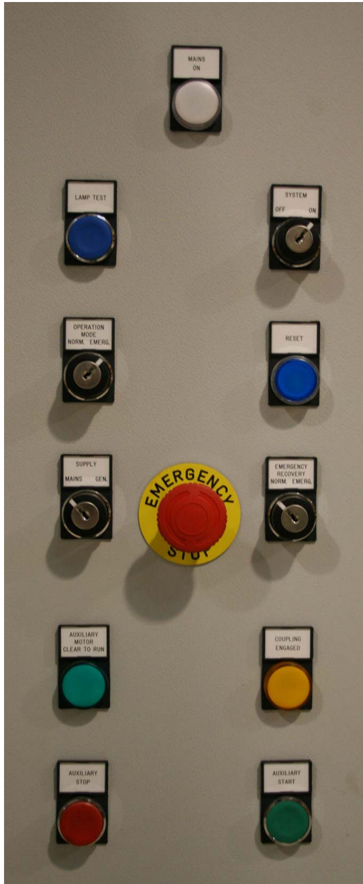
Figure 7: Winch Control Panel
