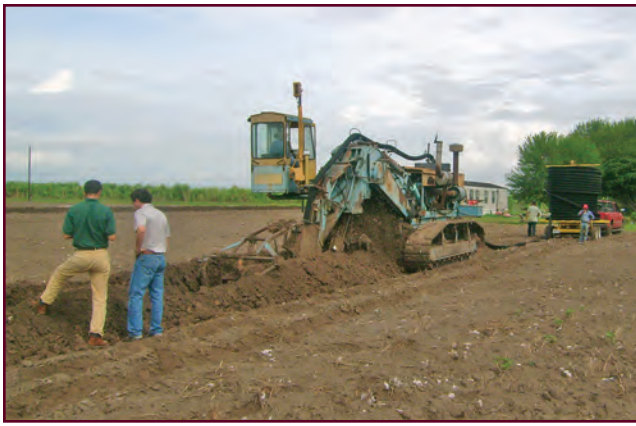
Figure 12. The machine unrolls the polyethylene pipe as it is laid into the soil by the trencher.
