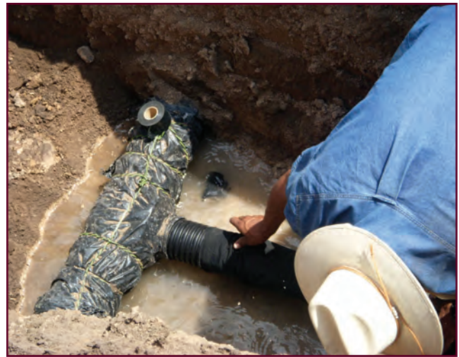
Figure 15. The interceptor drain is connected to the collector drain.
