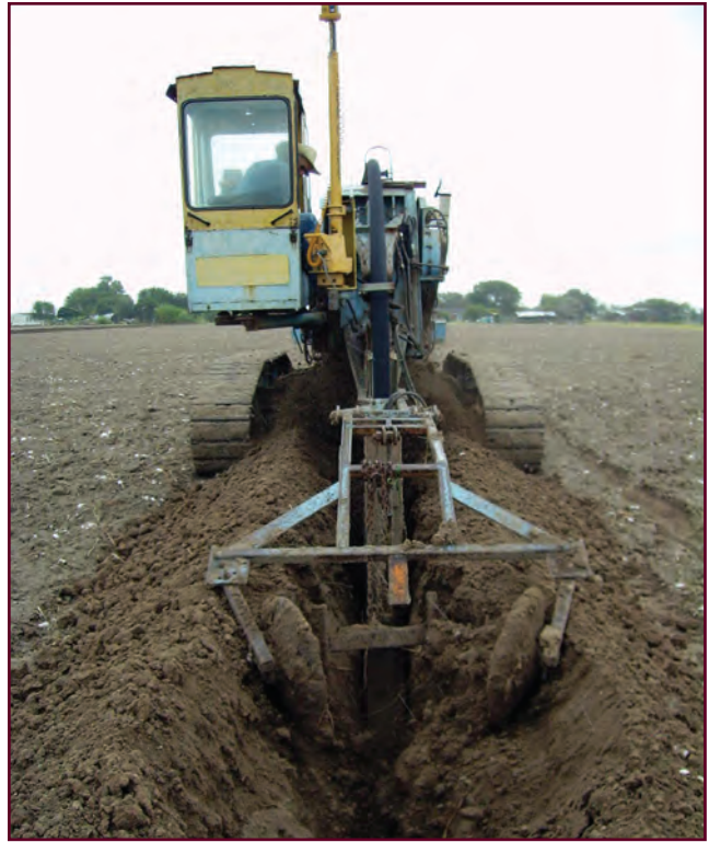
Figure 10. A trenching machine is used to install an interceptor drain lateral. The two disks help backfill the trench.
