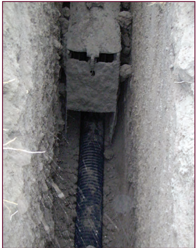
Figure 11. The interceptor drain lateral is placed at the bottom of the trench.
