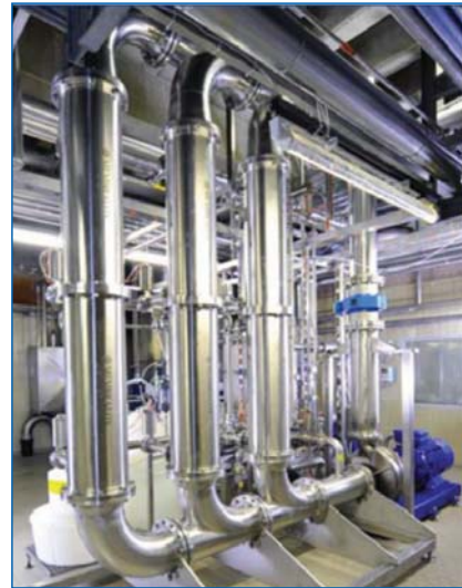
Figure 10d: Membralox Fermenter Broth Clarification System
