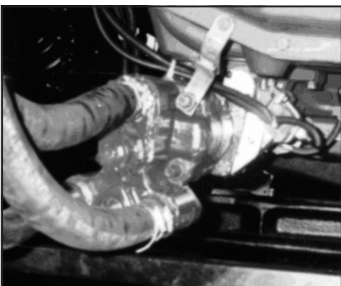
Improper Bracket Installation
