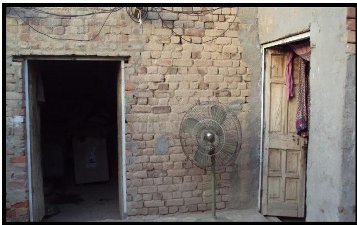
Photo 4.8: Recent addition of a room, only half is finished with cement
