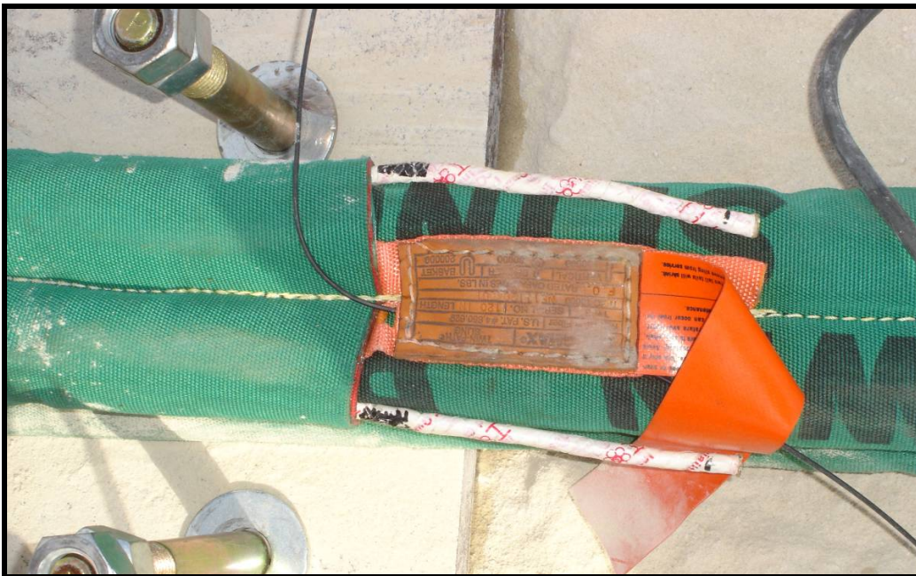
Figure 6. Check Tell-Tales and Fiber Optic Lines.
