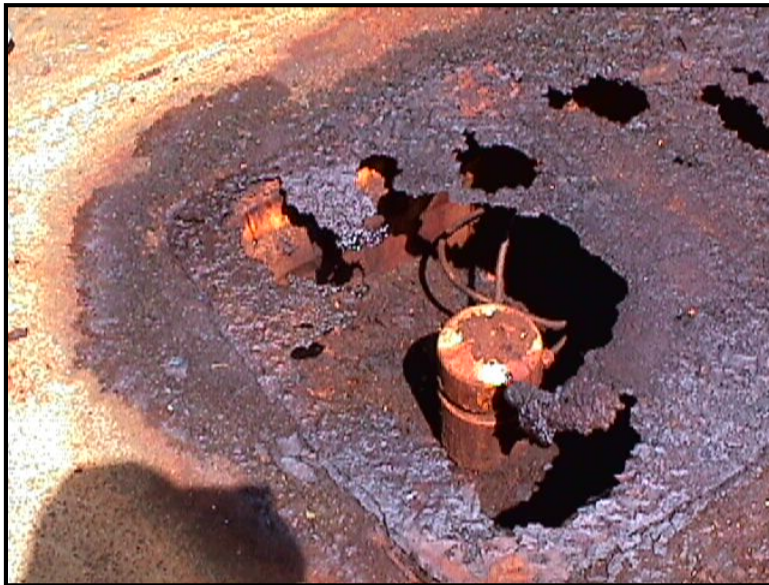
Figure B-24 Severe Corrosion of Cast Iron Cover on the Anode Well Head Box Caused By Chlorine Gas Vented into the Box.
