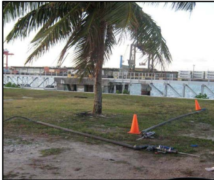
Figure B-17 Pre-Assembled Conduit System, Probe, and PRC for Submerged Use.
