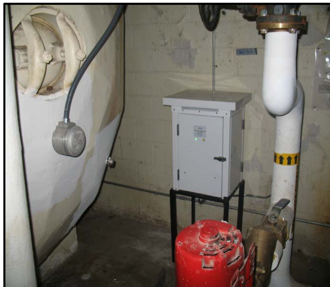
Figure B-35 CP System Rectifier and Anode Condulet Fitting on Side of Water Tank.
