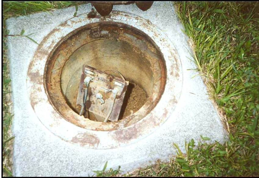
Figure B-9 Flush Mounted Current-Potential Test Station
