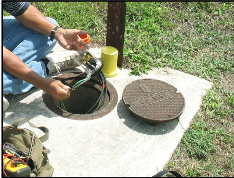
Figure B-6 Typical Ground Flush Mount Test Station
