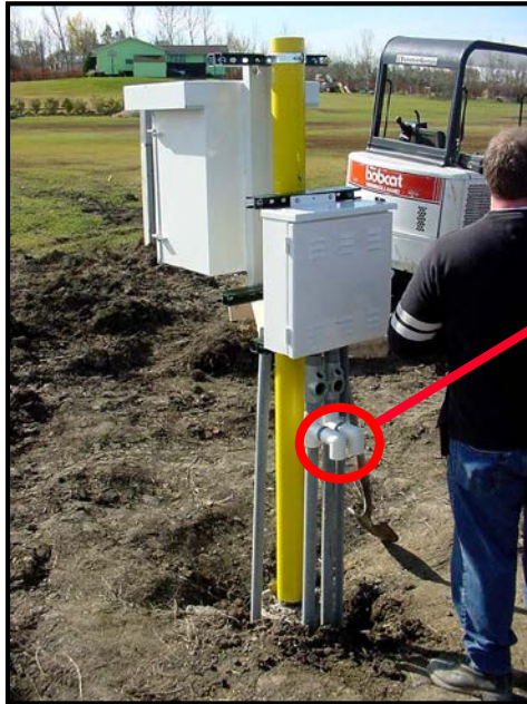
Figure B-23 Anode Column Vent Pipes Run Outside of Anode Junction Box.
