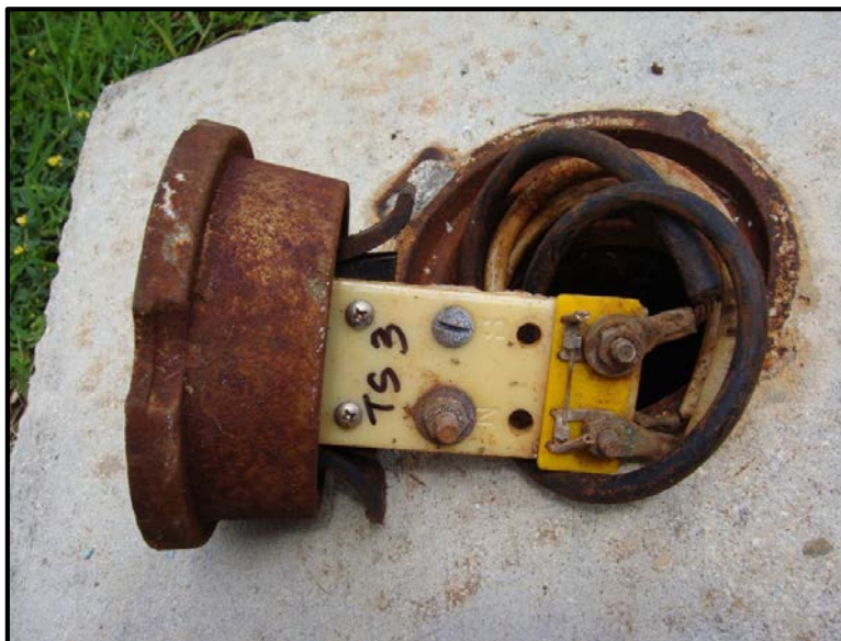
Figure B-14 Small Flush Mounted Test Station with Too Many Large Sized Wires.
