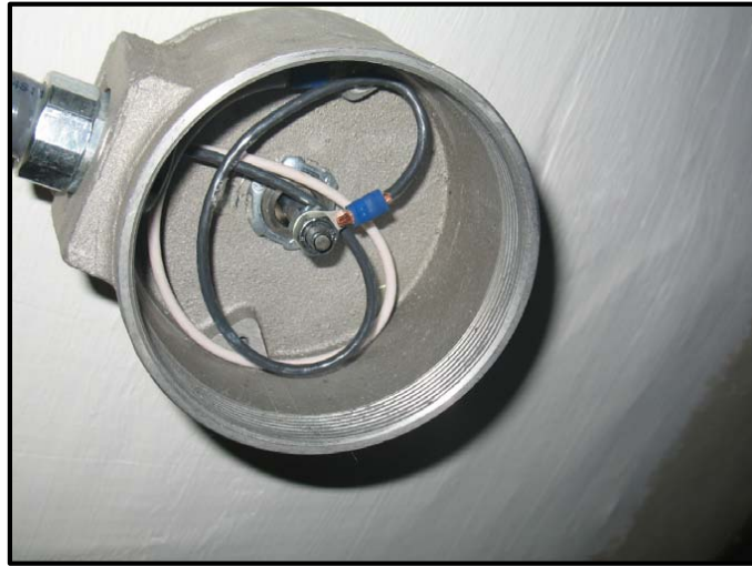
Figure B-36 Close up of Condulet Fitting Showing Anode Rod Extending Out of the Storage Tank.
