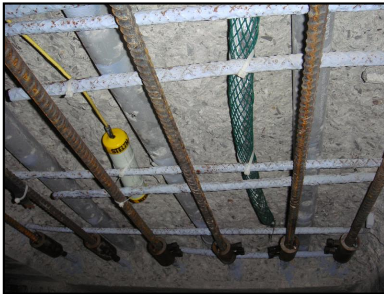
Figure B-27 Discrete Zinc Anode (Wrapped in Green Mesh) in Concrete Deck Repair. Device with the Yellow Lead Wire is a Permanent Reference Electrode.
