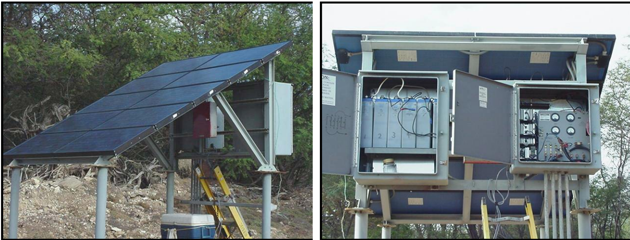
Figure 4-2 Small Solar Powered CP System. Solar Panels Shown in Picture on Left. Battery Bank and Control Center Shown on Right.
