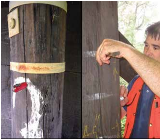
Figure 2.3—Probes are used to assess depth of cracks, checks, and through splits in timber bridge elements.
