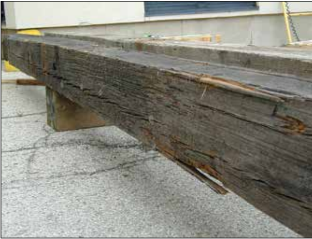
Surface decay and multiple cracks
