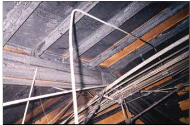
Figure 5.4—Charred and uncharred wood members in the Building 2 fire at the Forest Products Laboratory.
