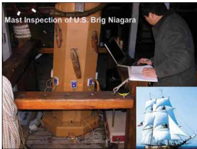
Figure 4.5—Inspection of the masts of the U.S. Brig Niagara using acoustic tomography.
