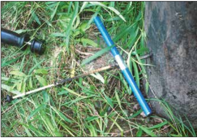
Figure 2.8—An increment core can be used to conduct inspections of timber bridge elements. This image shows an extracted core from an in-service timber pile ready for examination.
