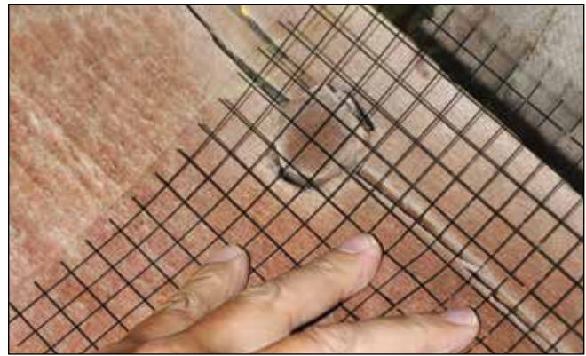
Figure 6.6—Example of using grid to establish the size of knot in bridge member. The measured knot in the example is 1-1/2 in.
