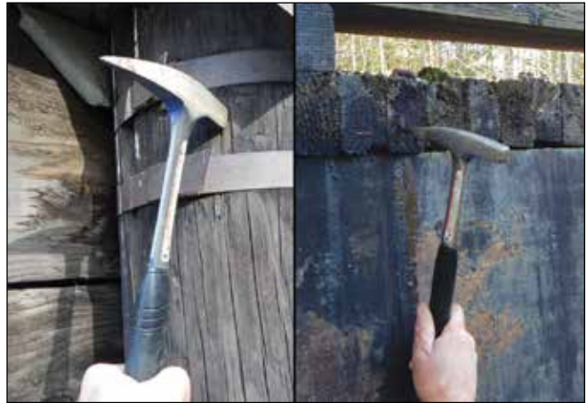
Figure 2.1—A hammer pick is an effective tool for initial assessments of timber bridge elements.
