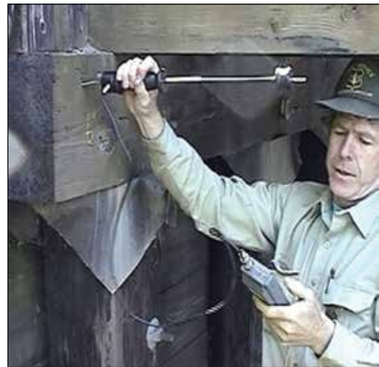
Figure 2.7—A pin-style moisture meter is used to determine moisture content of timber elements.
