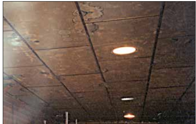
Figure 1.6—The ceiling panels were stained and discolored.
