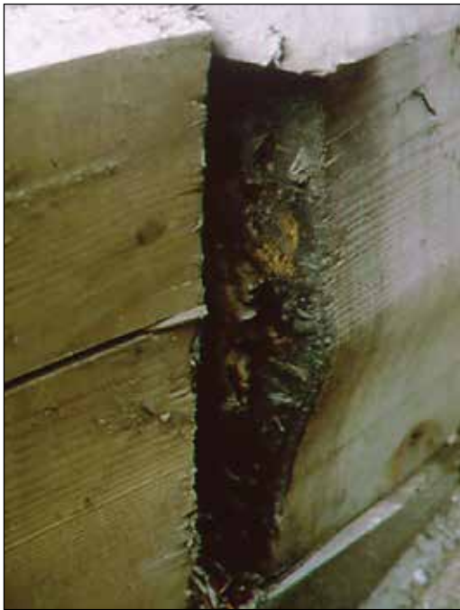
Figure 1.4—The timber beam's outer shell buckled as a result of interior deterioration.
