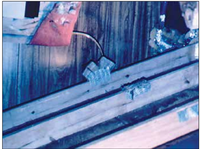
Figure 1.11 —Metal plate connectors were cut and bent so that the webs could be removed. This should never be done.
