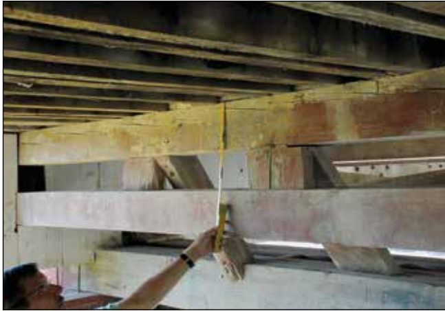
Figure 6.8—Example of using checking in a member to measuring the slope of grain in bridge. The end of the scale points to the start of one check.
