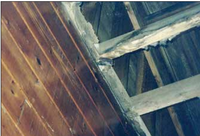
Figure 1.9 —As a consequence of the moisture exposure, wood members in the roof and walls also contained areas of deterioration.
