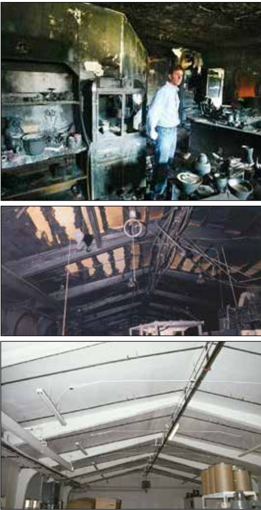
Figure 5.10—Post-fire inspection (top) of residence; post-fire (middle) and post-repair (bottom) of Building 2 at the Forest Products Laboratory. Top photo courtesy Montana Standard; www.mtstandard.com .
