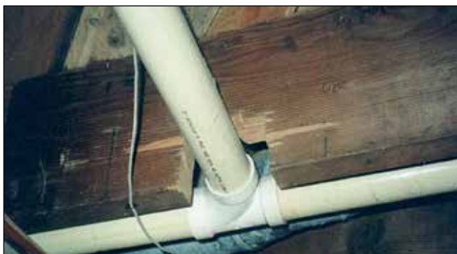
Figure 1.14 —A floor joist was cut to make room for plumbing. This should never be done.
