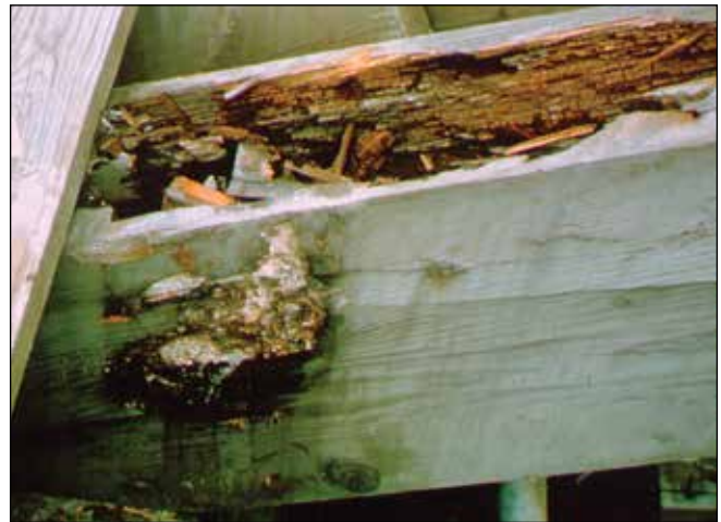
Figure 1.2—Fruiting bodies can indicate extensive damage inside the beam.
