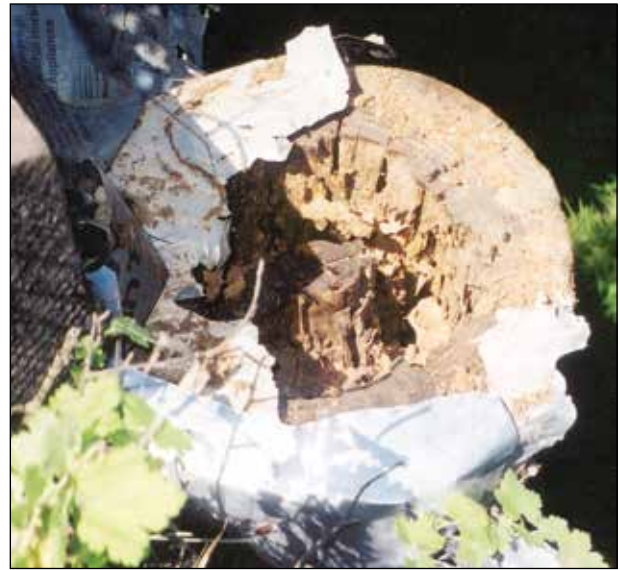
Figure 1.10 —Damage to a bridge piling.
