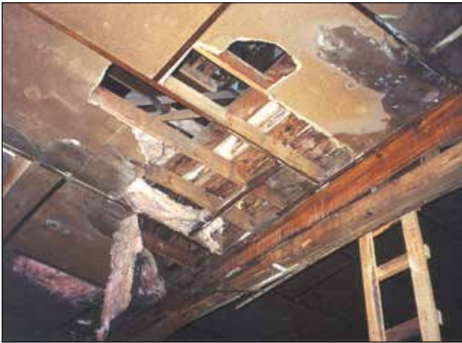
Figure 1.8 —Removing the ceiling panels revealed that the fiberglass insulation was saturated with water.
