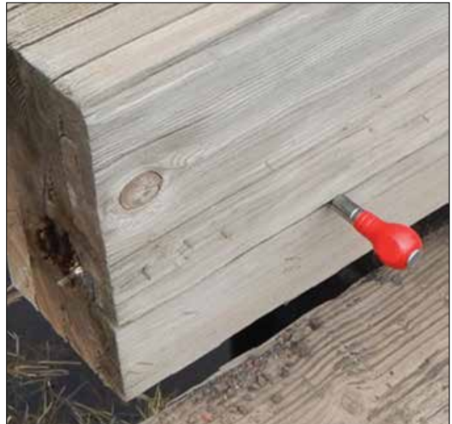
Figure 2.2—An awl is used to assess depth and presence of decay in a horizontal split.
