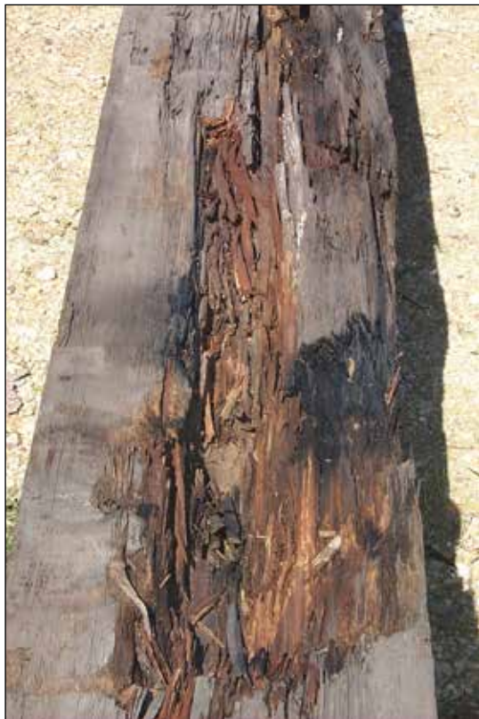
Severe decay damage
