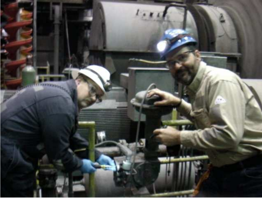
BTC Instrumentation grads Micah and Mark working on a control valve near an ore crushing mill in Alaska.
