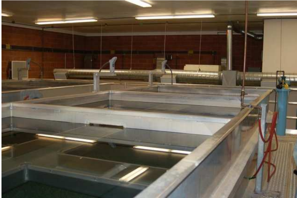
Potable water filtering at the city of Arlington, Washington.
