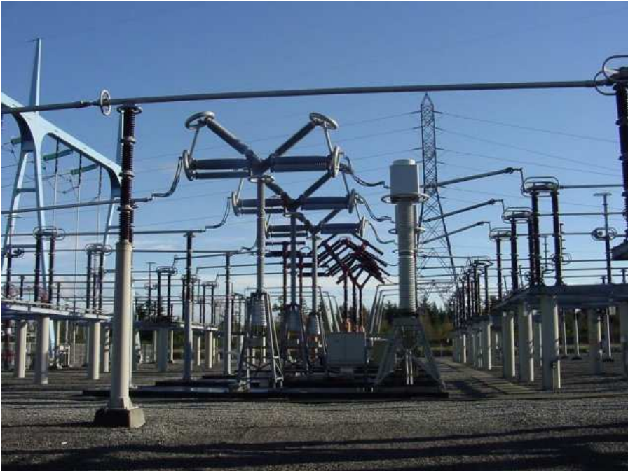
Bonneville Power Administration's Custer, Washington substation switchyard (500,000 volts).
