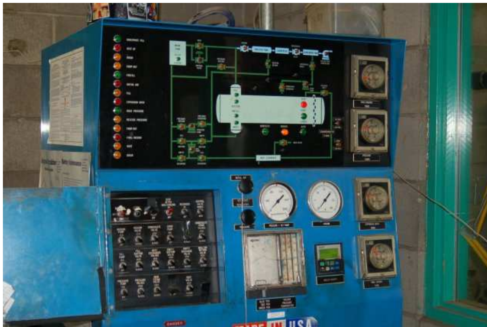
A retort used to pressure-treat lumber.
