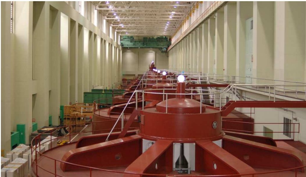
Hydroelectric turbine generators at Grand Coulee Dam in Washington.
