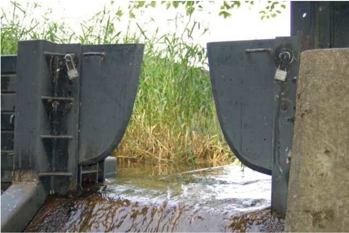
A Sutro weir used to measure the flow of water out of lake Padden in Bellingham, Washington.
