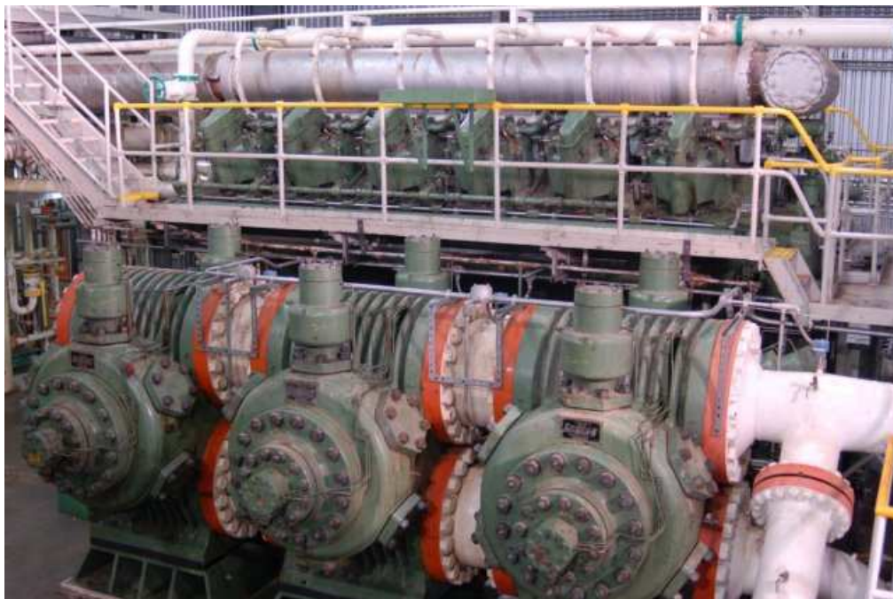
Large reciprocating (piston) engine used to compress natural gas.
