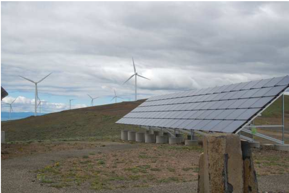
Photovoltaic array at the Wild Horse wind farm near Ellensburg, Washington.
