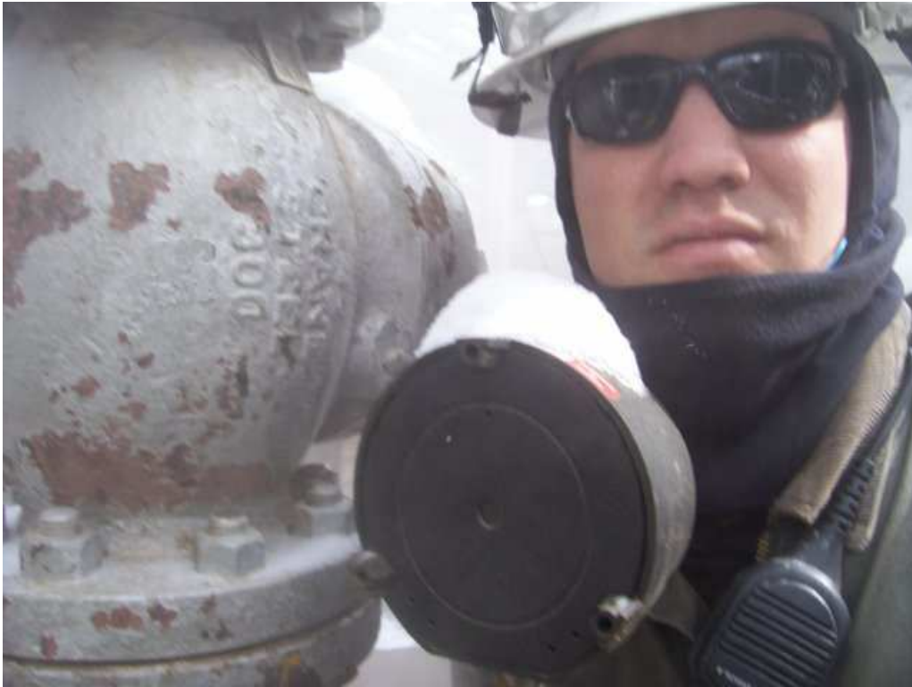
BTC Instrumentation grad Corey services a control valve at a Wyoming oil refinery during a winter shutdown.
