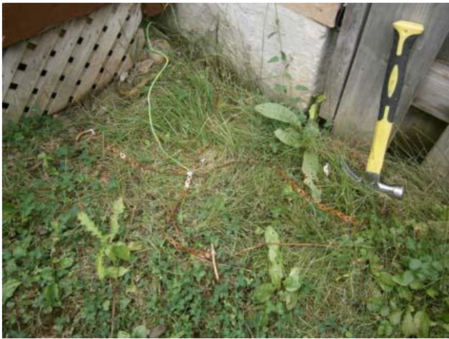
Figure 12 Grounding at the Antenna
