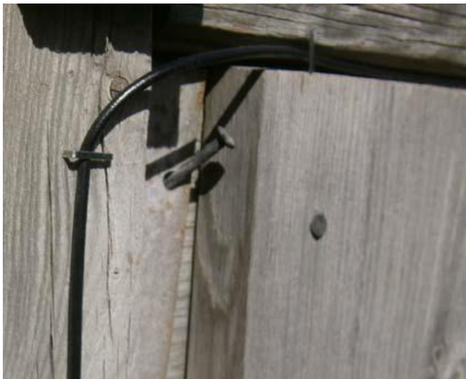
Figure 13 Staped Wire of Beverage Antenna
