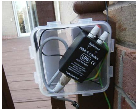
Figure 15 Transformer of Beverage Antenna in Open Plastic Food Box
