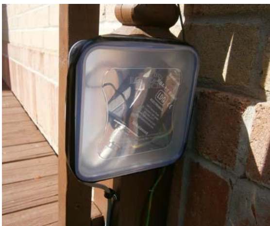
Figure 17 Transformer of Beverage Antenna in Closed Plastic Food Box
