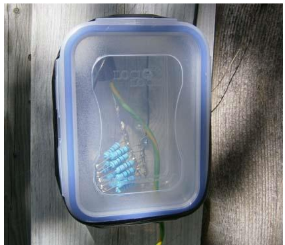
Figure 16 Termination Resistor of Beverage Antenna in Closed Plastic Food Box
