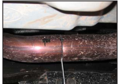
#4 Cut at Bottom of Down Pipe
