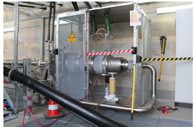
Figure 7 On site partial discharge measurement
