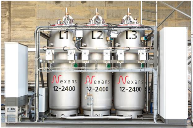
Figure 3 Fault current limiter delivered on site in Essen
