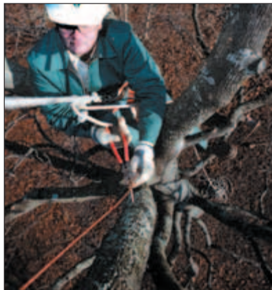
Closing drive fastener: The conductor is installed starting near the top of the tree. From this point downward the conductor is fastened to the tree with drive fasteners.
