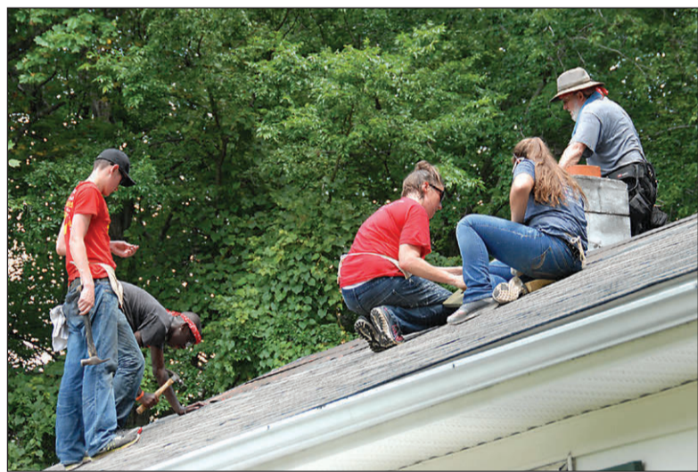
Volunteers with Impact Virginia made the area a better place through their week-long mission to repair houses for the needy. Above, a roof is replaced on a home near Urbana.
