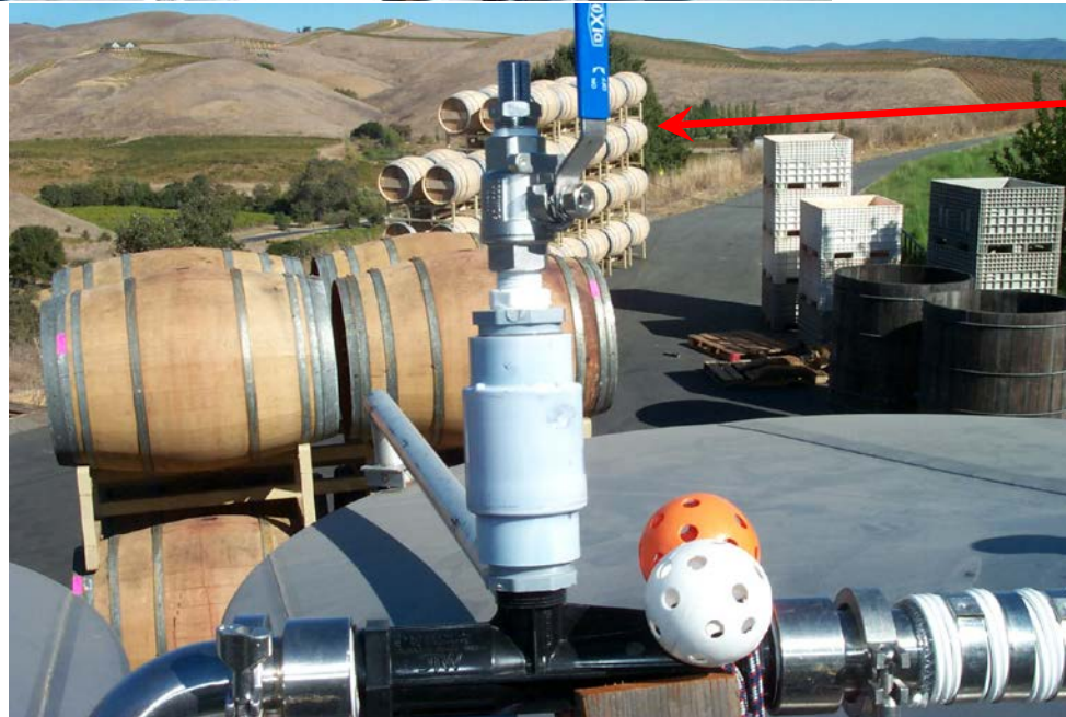
Note shut-off valve
