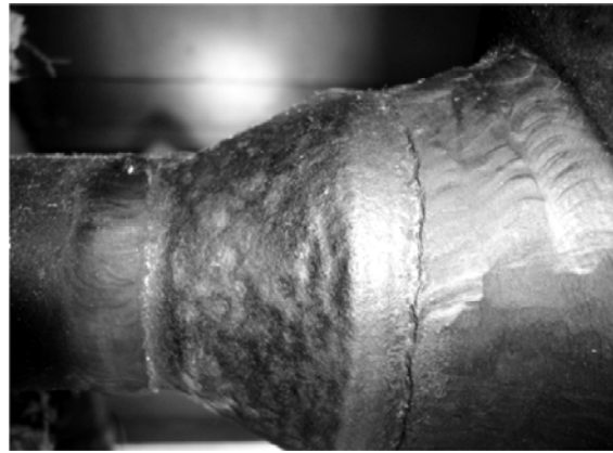
Photograph No. 02: Pitting marks and general surface grooving (1.5 mm deep) noticed on external surface of weldolet.
