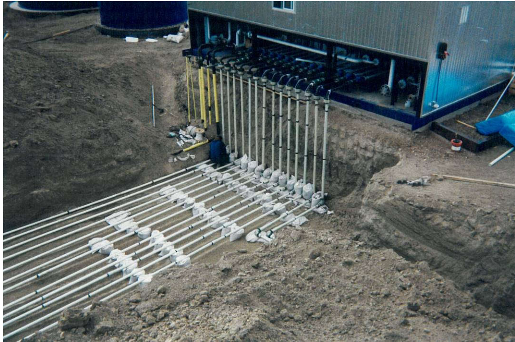
Figure 4-1 Pipeline Riser showing use of Sand Bagging for Support and Thrust Blocking. Composite Riser Extends above Grade to Flange Transition to Steel Piping (Photo used courtesy of Western Fiberglass Pipe Sales Ltd)
