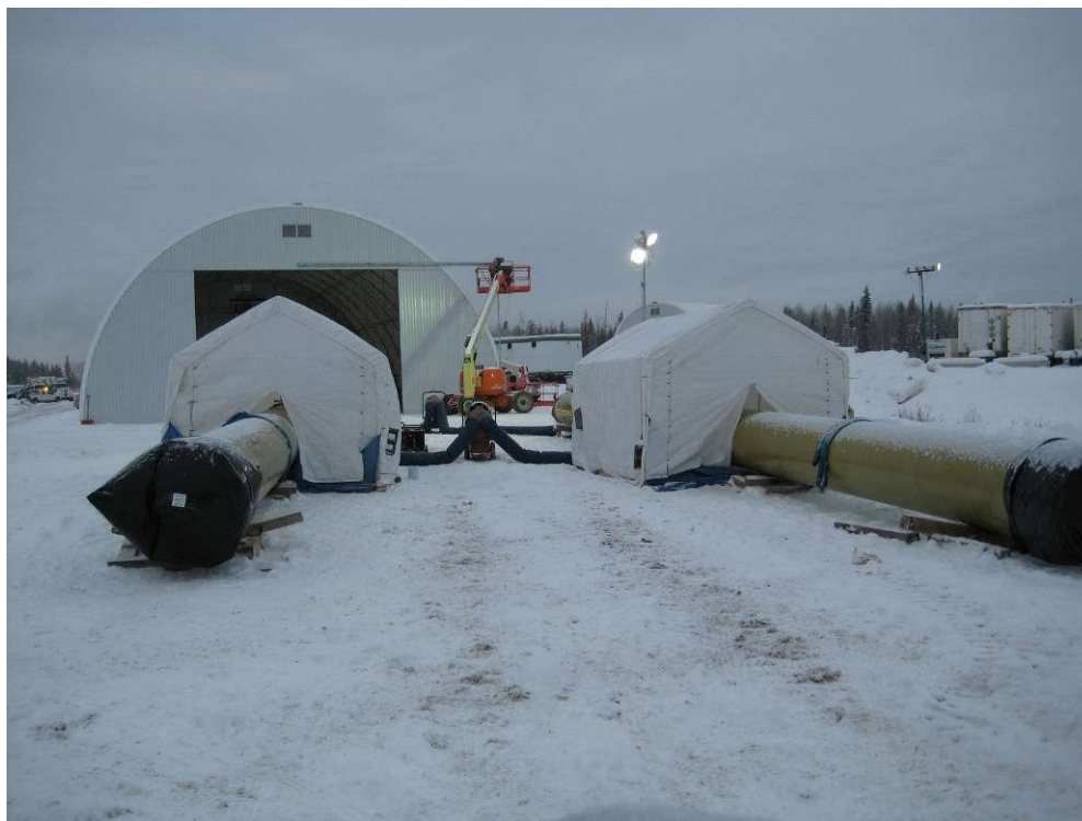
Figure 8-1 Provision of Shelters for Joining Composite Pipe; (Photograph courtesy of Fiber Glass Systems and Fiberglass Solutions Inc)
