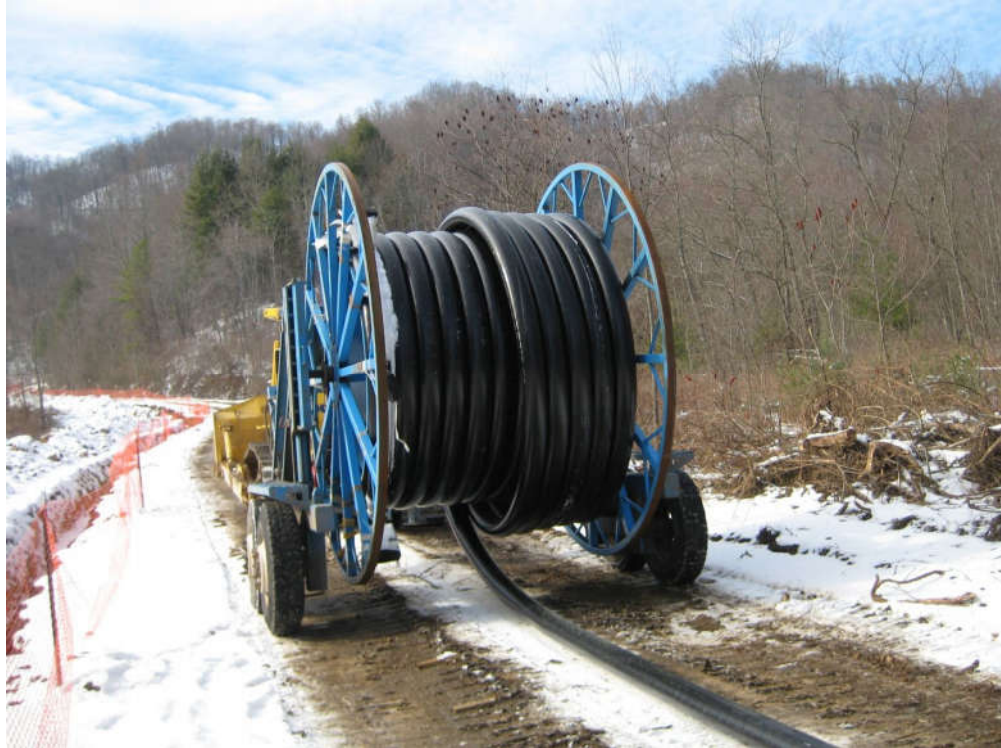
Figure 7-3 Spoolable Pipe Transport on Reel Trailer (Photograph courtesy of FlexSteel Pipeline Technologies Ltd.)
