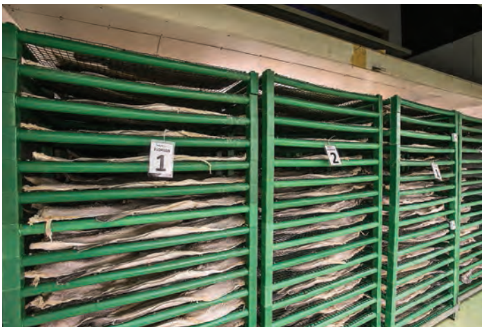
PHOTO 3 Fish drying in a geothermal tunnel dryer in Iceland
