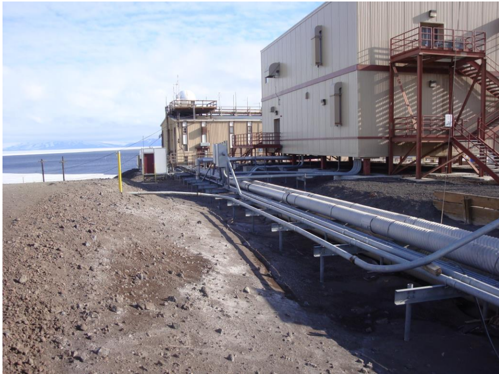
Utilidor looking SW with Building 189 (JSOC) in the foreground and Building 165 (MAC OPS) in the background
