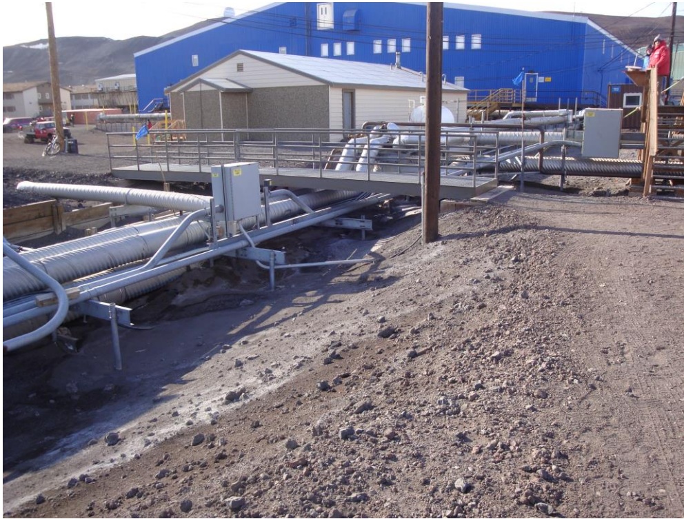
Utilidor looking north with Building 107 (Southern Exposure) and Building 155 in the background
