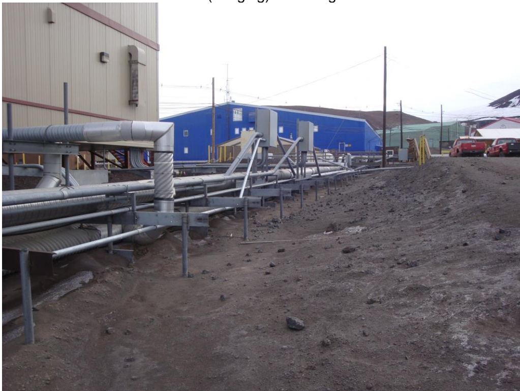
Utilidor east of Building 189 (JSOC) looking northeast at Building 155
