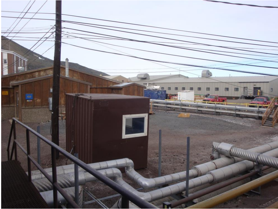
Looking SE from south platform of Building 155 with Building 108 (Gallagher's) and Building 001 (Crary Lab) in the background
