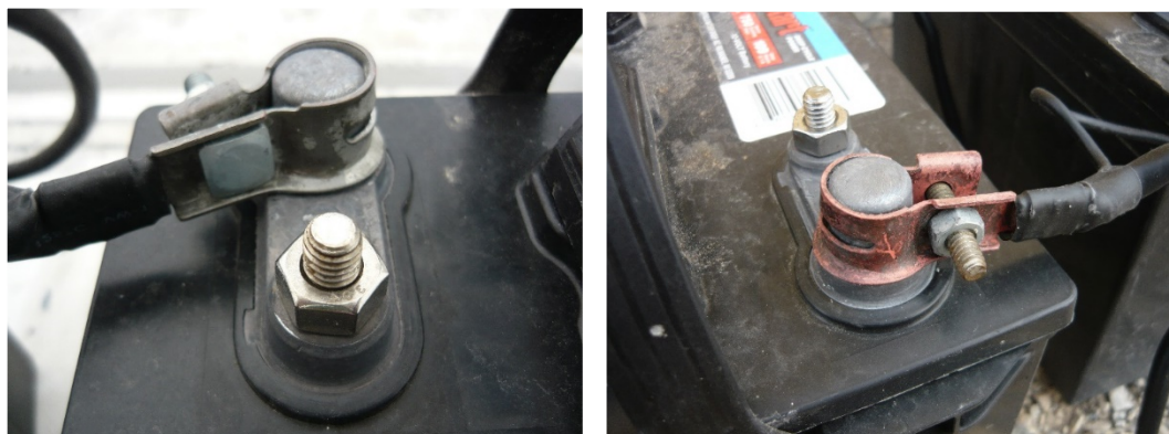
Figure 19a. Before exposure (left) and after one exposure (right). Notice the immediate corrosion.
