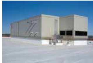
Packaged Rooftop Units
