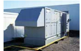
Energy Recovery Units
