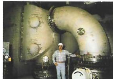
A 166,000 sq.ft. steam surface Condenser.
