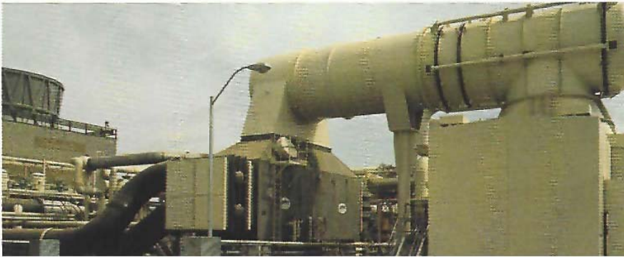
A 54,000 sq. ft. steam surface condenser for 32 MW geothermal power plant in California.
