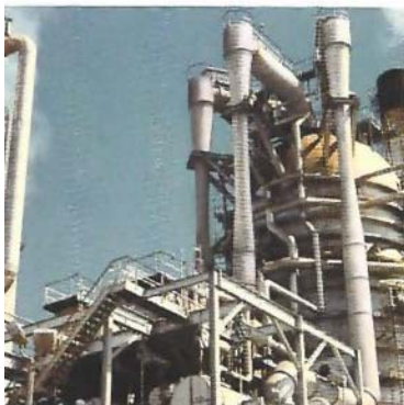
Triple element booster Ejectors in refinery service.
