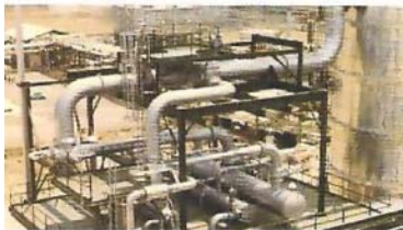
Ejectors in vacuum distillation service.
