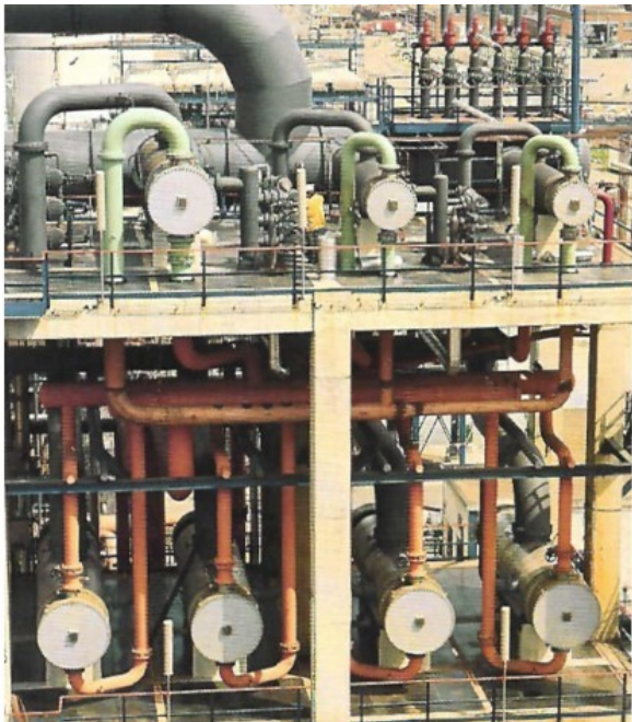
Shell and tube condensers in oil refinery vacuum service.
