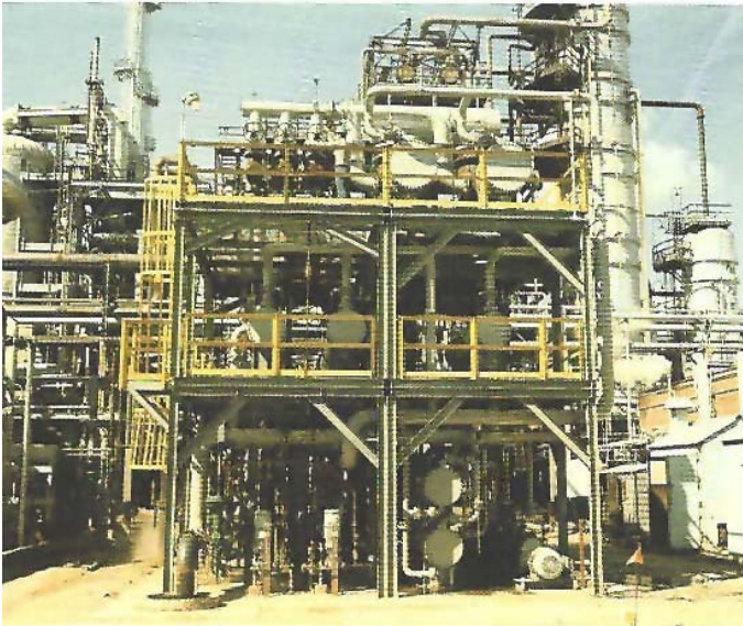
Six section modular combination ejector system-liquid ring vacuum pumps in refinery service.
