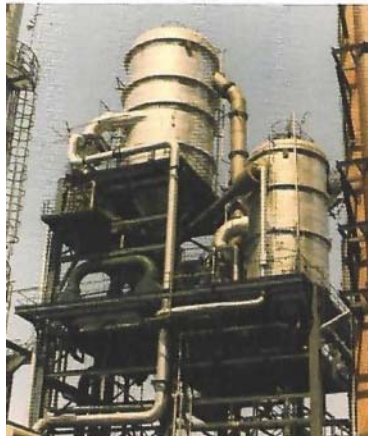
Ejector and Condensers in a urea plant.
