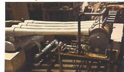
3,400 ton steam vacuum refrigeration unit.
