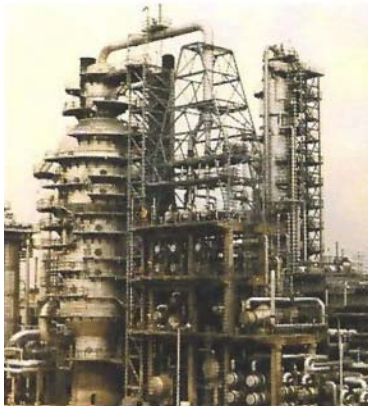
Three-stage Ejector system in refinery service.
