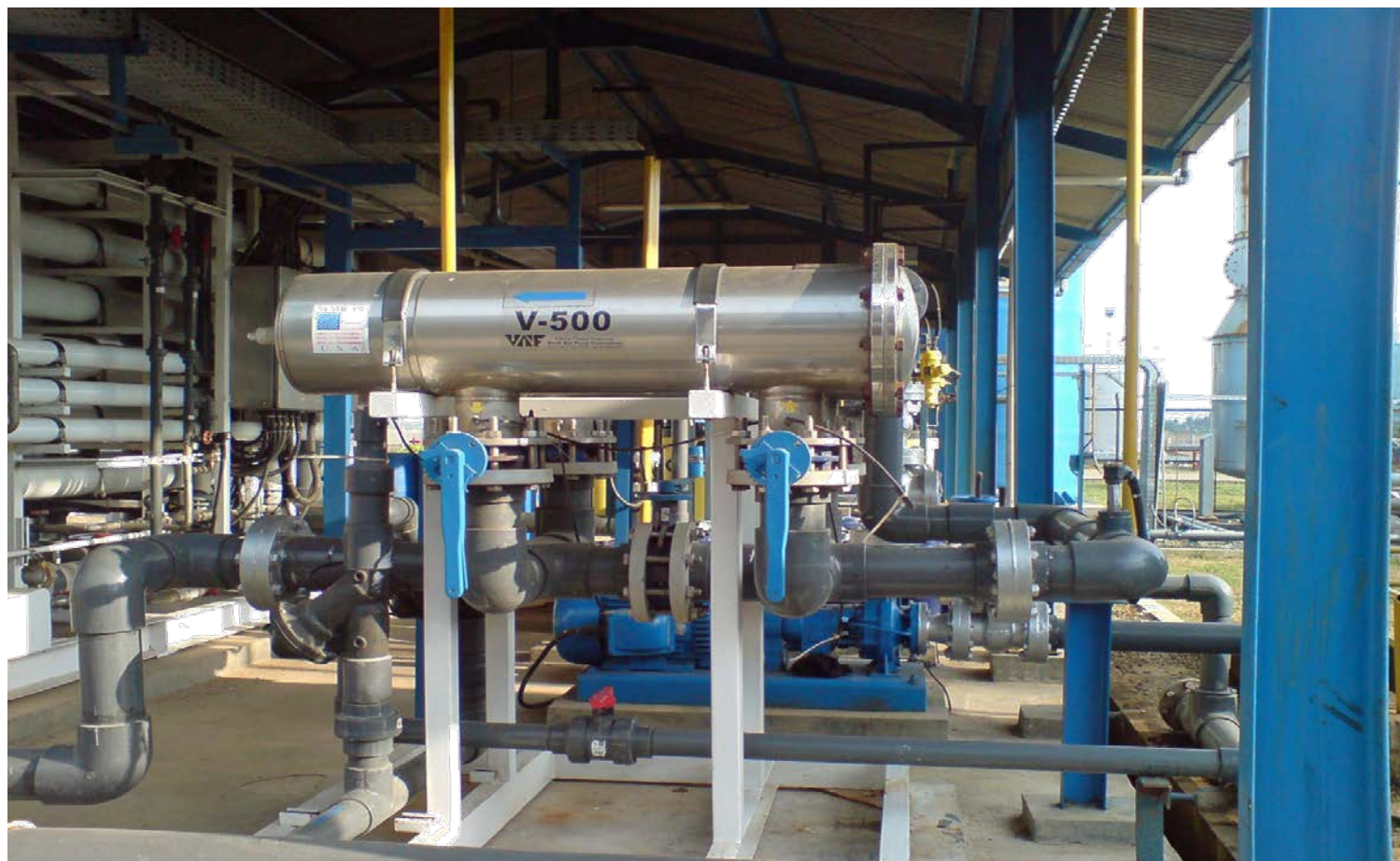
Oil and Gas Company - Bakasi, Indonesia Two V-500s 25 micron 45 m 3 /hr (200 gpm) each Pre-Filter RO
