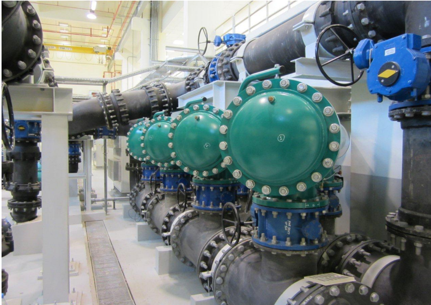
University – Riyadh, Saudi Arabia 1,100 m 3 /hr (5,000 gpm) Well/Municipal Water – Landscape Irrigation
