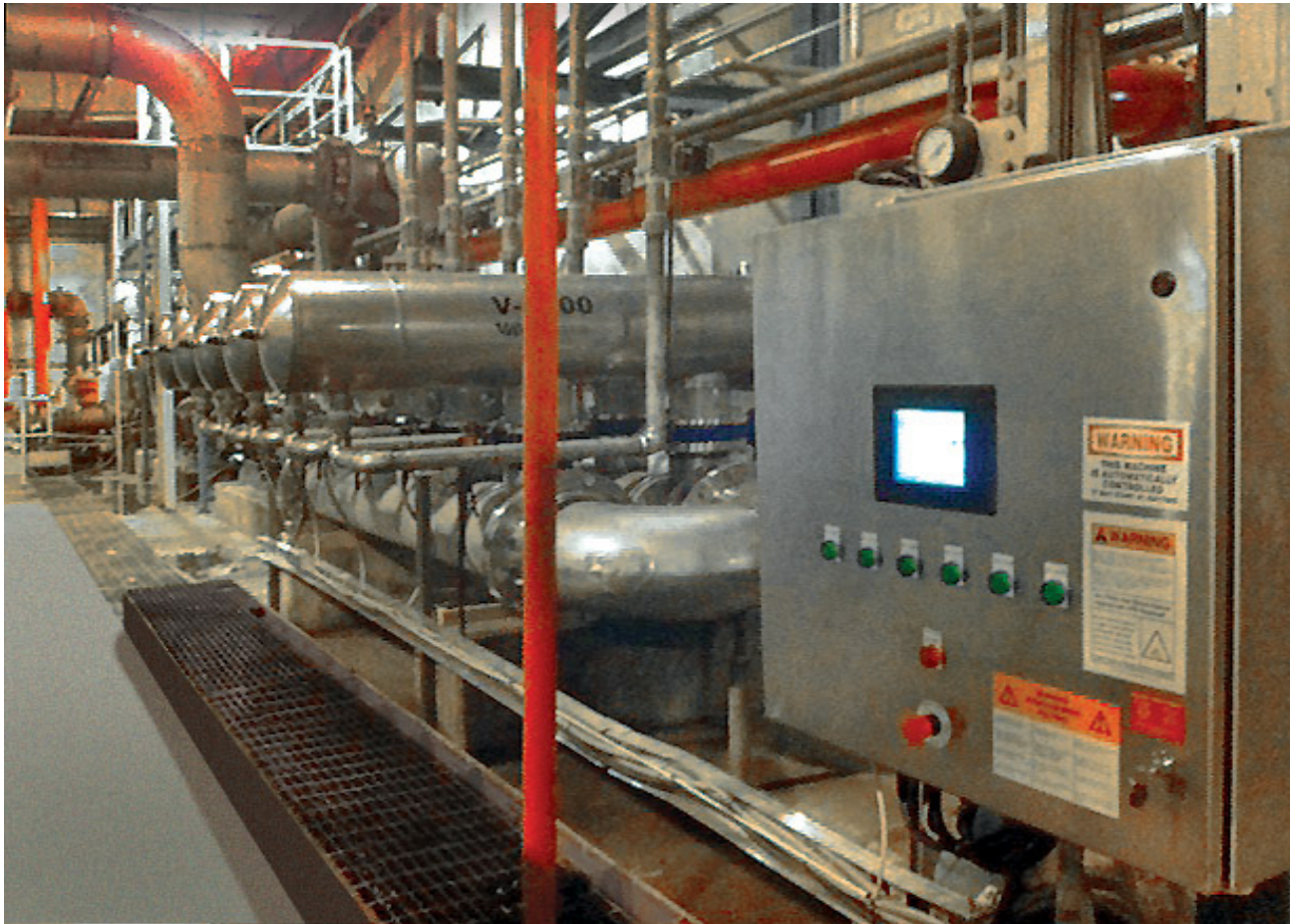
Irving Tissue Paper Plant – Dieppe, New Brunswick, Canada Five V-1500s 80 micron 454 m 3 /hr (2,000 gpm) Intake Water
