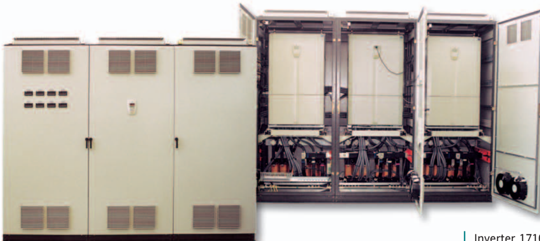
Inverter 1710 A, controlling a 1300kW-Motor.
