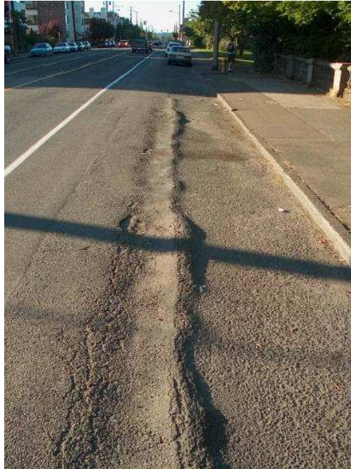
Figure 2 Rutting on the road surface
