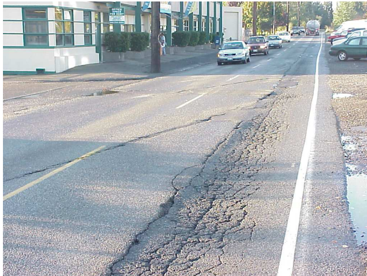
Figure 3 Fatigue cracking and rutting on the road surface
