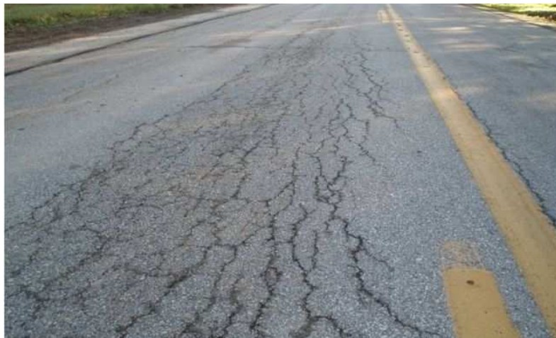
Figure 1 Fatigue cracking on the road surface
