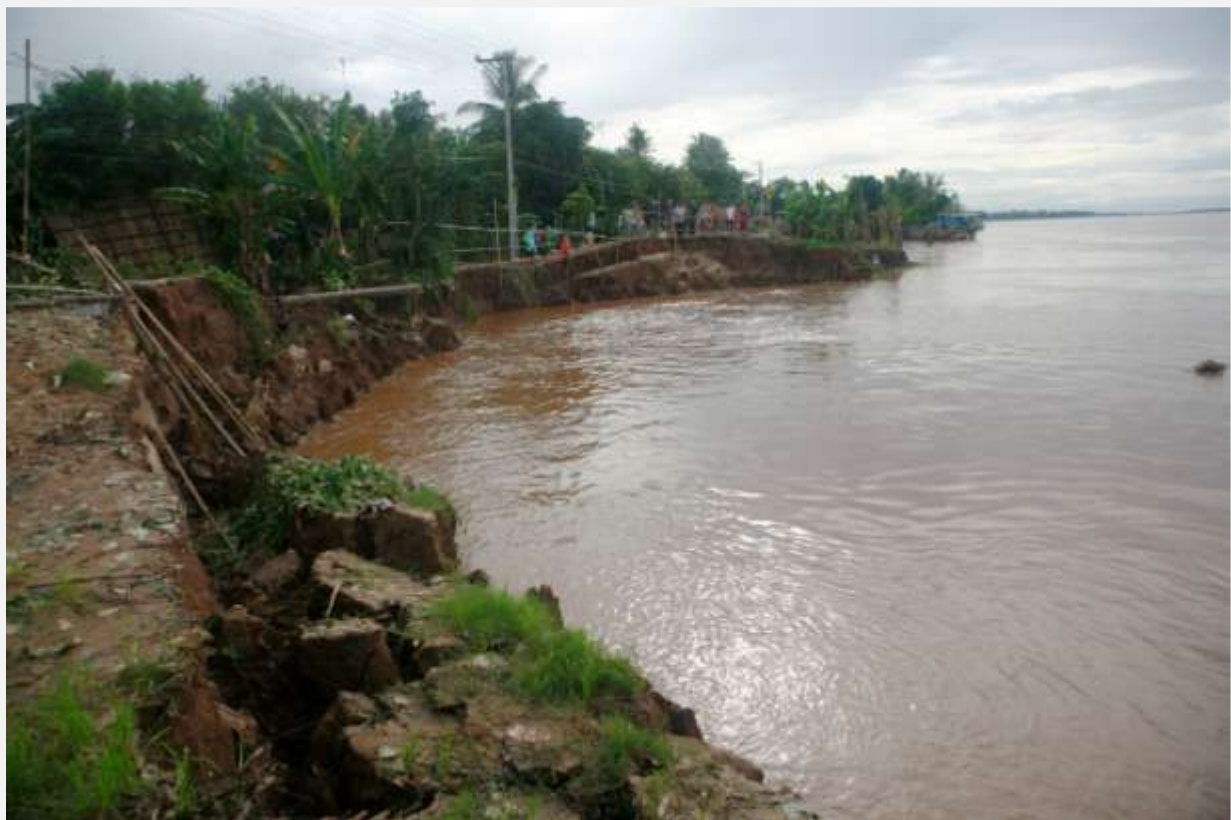
River bank erosion is becoming more acute with heavier peak flow
