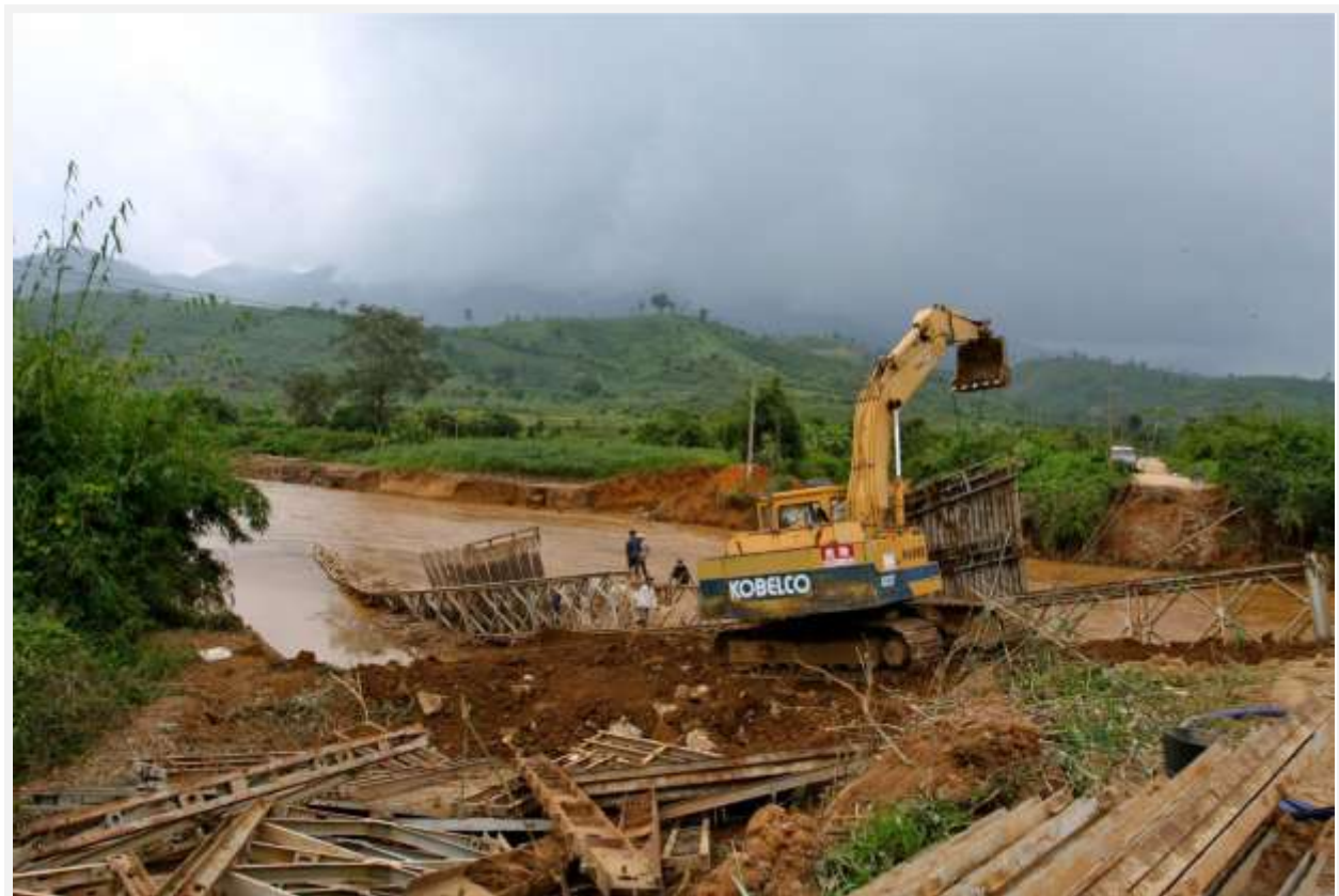
The bridge linking Dak Tram commune and other communes (Kon Tum Province) was destroyed by Typhoon Ketsana (2009) 29
