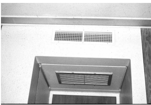
Figure 70. Supply and return grilles for a concealed fan-coil unit.
