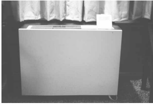
Figure 55. A unitary air-conditioning unit in a motel room.
