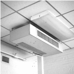
Figure 69. A horizontally-oriented fan-coil unit.
