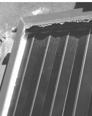
Figure 19. Active solar collector.
