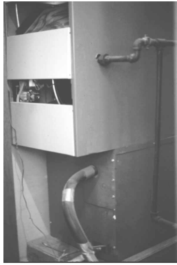
Figure 12. Exterior view of a gas furnace.
