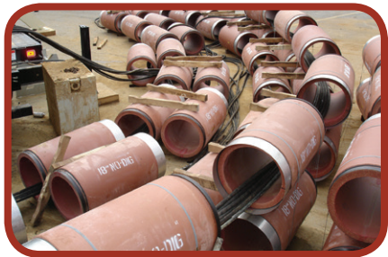
Figure 38: Jacking pipes staged at the launch pit on a pilot tube project utilizing a powered cutter head.
