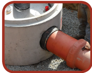
Figure 33: Two points of flexibility at this manhole are provided by the flexible manhole connector and the flexible compression joint on the short length of pipe.
