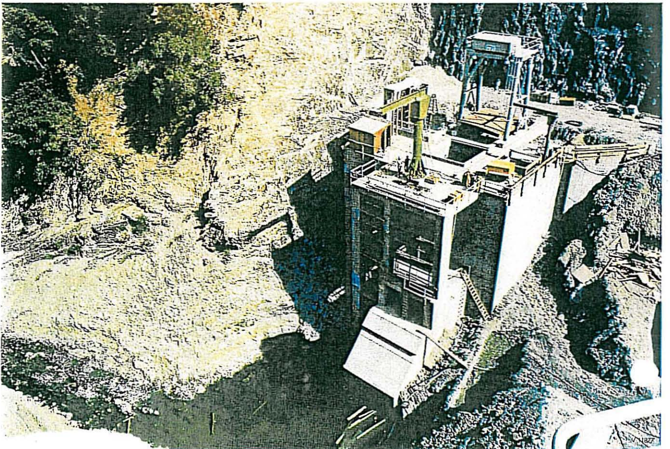
Fig. 30 Oxbow Power Station nearing completion. The cover closing off the opening for the installation of the generator rotor has been lifted by the crane.
