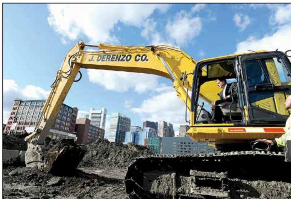
Mayor Walsh used an excavator to ceremonially kick off construction for One Seaport Square on Nov. 14, 2014. Mayor’s Office photo by Don Harney
