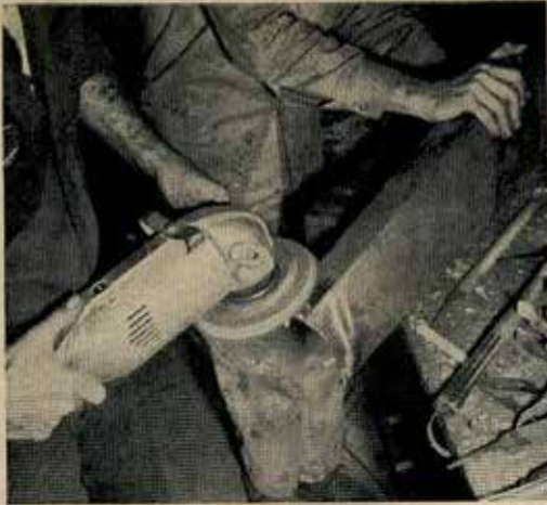
17 Using a 36 close-coat grinding disc and electric grinder, smooth out areas around welded studs on the straight bars.
