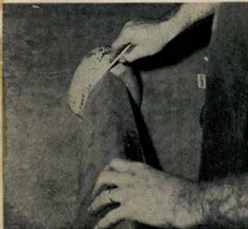
13 Now we are ready to attach light shell to grille bar; mark location of holes on the light shell to be drilled for attachment.
