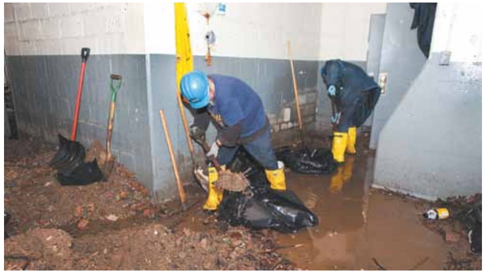
NYCHA staff shovel out the sludge left behind by the flood water at Red Hook East in Brooklyn on November 5.
