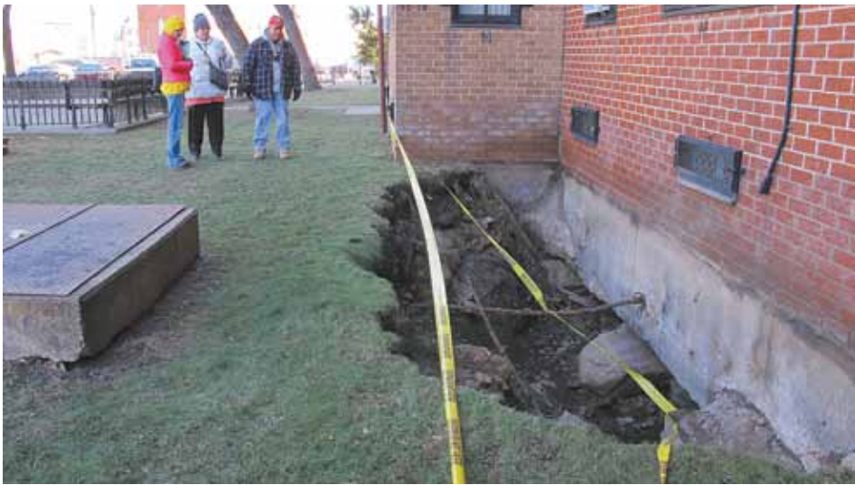
Many buildings damaged by the storm had sink holes that allowed water to flow under the structure, such as at Carleton Manor, shown on November 3.
