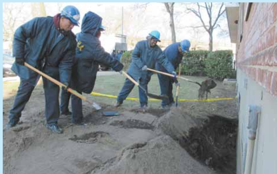
NYCHA staff work on repairing damage caused by Hurricane Sandy at Hammel Houses in Queens on November 3, 2012.
