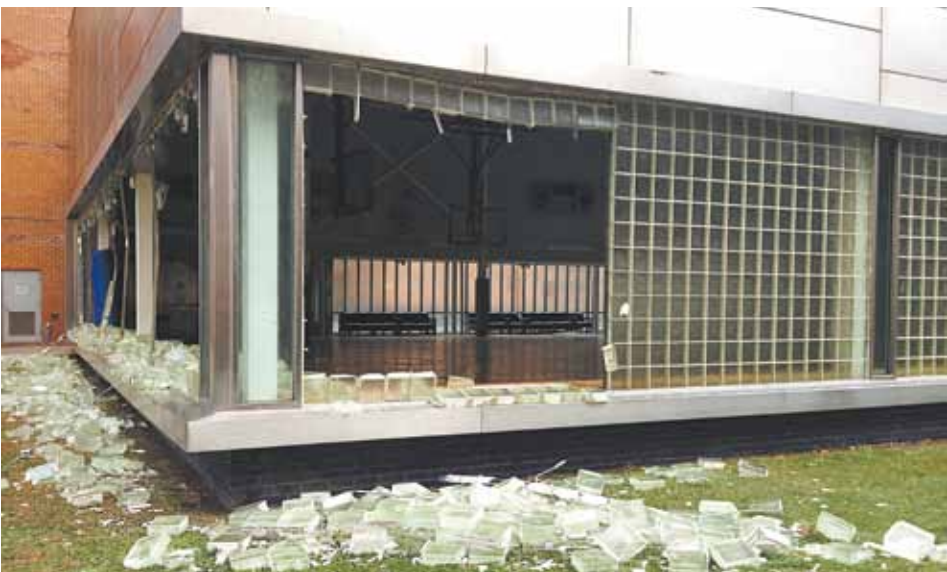
Damage to the Hammel Houses Community Center in Queens on October 30. Photo by Gina Tutt.
