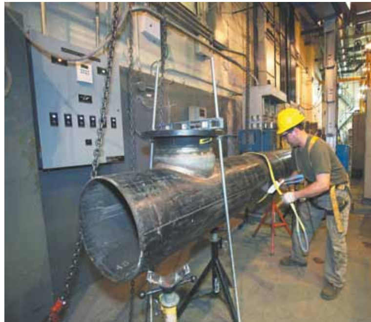
Among the projects that will be completed during the next six months using $69 million in capital funds is a new boiler system at Edenwald Houses in the Bronx.
