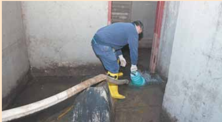
A NYCHA employee pumps water out of the basement at Red Hook West Houses on November 5, 2012.
