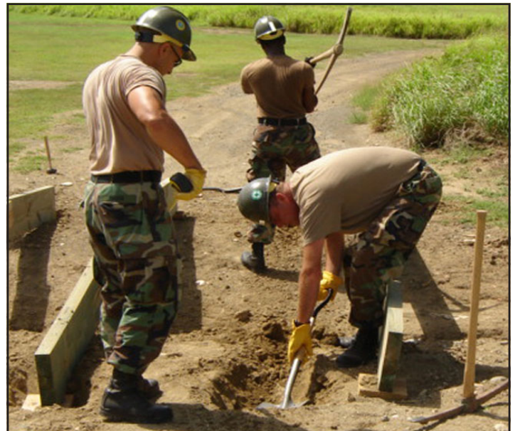
BUI(SCW) Freddy Pagan, SWCN Kenneth Collier, and CE1(SCW) Walter Gibbs dig the foundation for one of the bridges.
