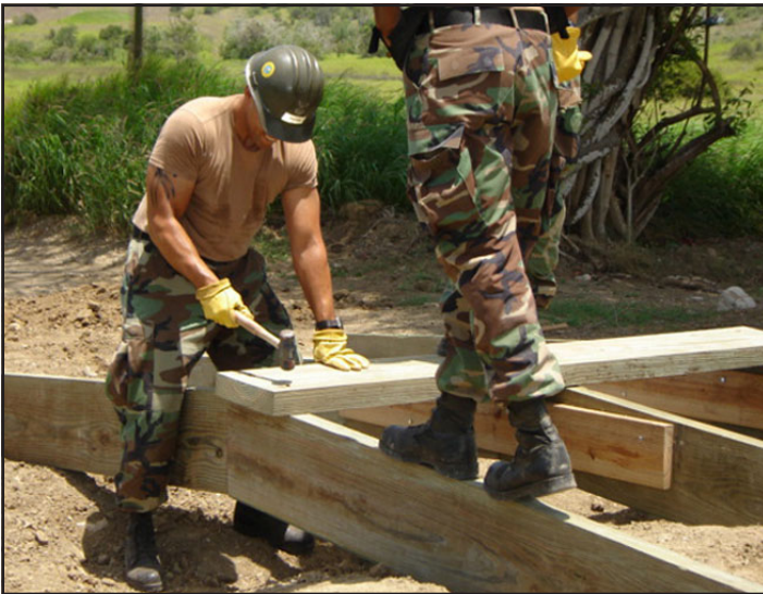
BUI(SCW) Freddy Pagan puts together framework for one of the four cart bridges built by Self-Help.
