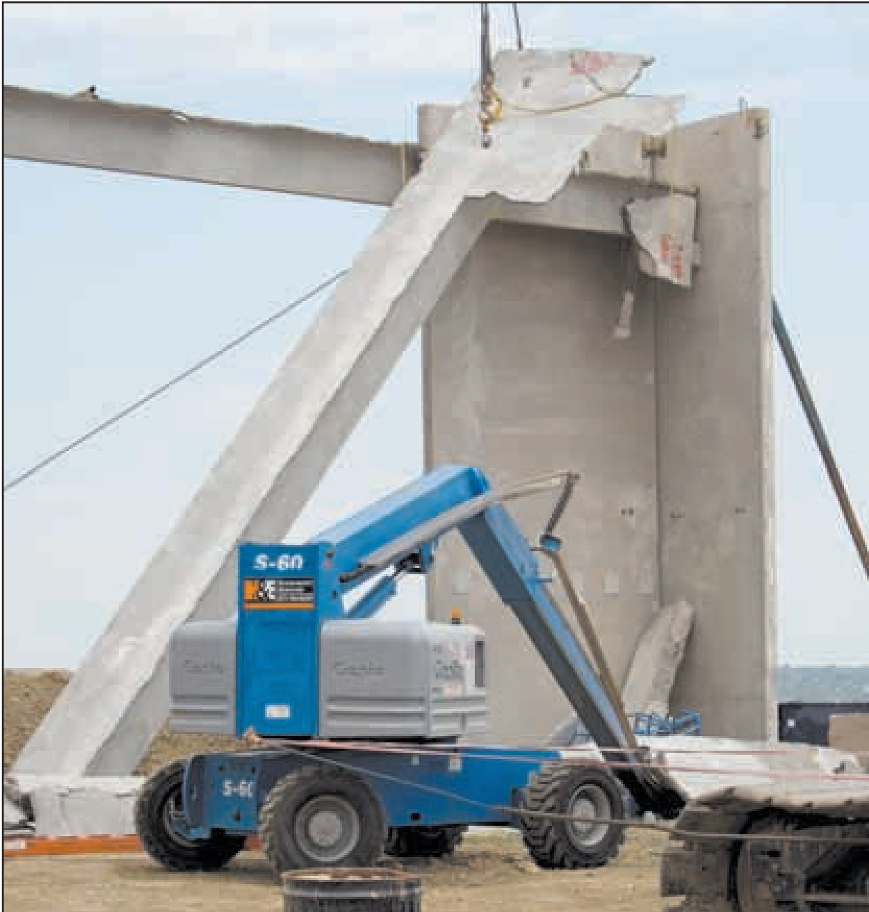
A concrete girder leans against a concrete wall after collapsing Monday at the site of a future 4th Brigade Combat Team, 4th Infantry Division operations center.
